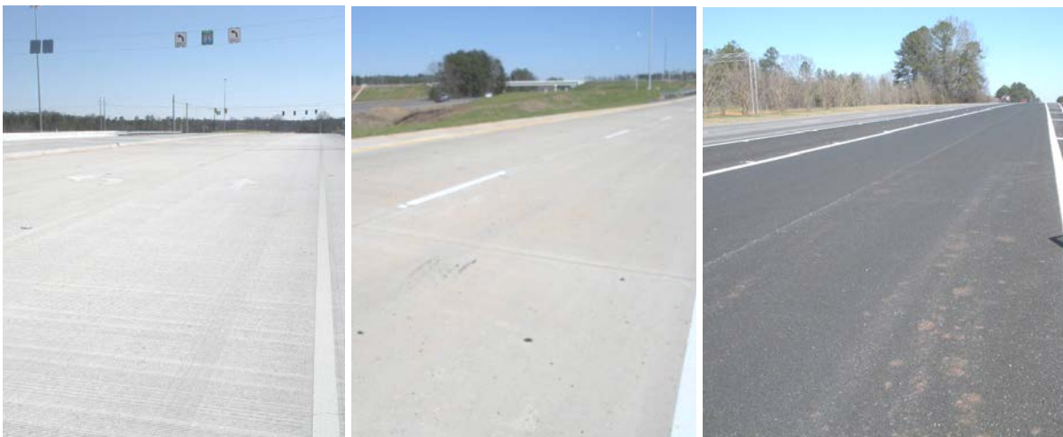
Figure 15. Newly constructed pavement test sections (left to right): Kia Boulevard bridge deck, Exit 6 off-ramp, and Exit 6 on-ramp.
