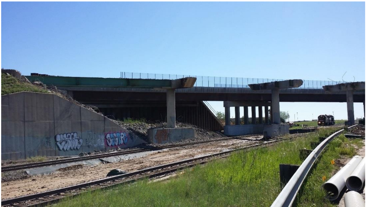
Figure 18. Photo. Old eastbound bridge being demolished, new bridge E-17-AEK in background, June 2015. E-17-AEK is in service at the time of this photograph.
