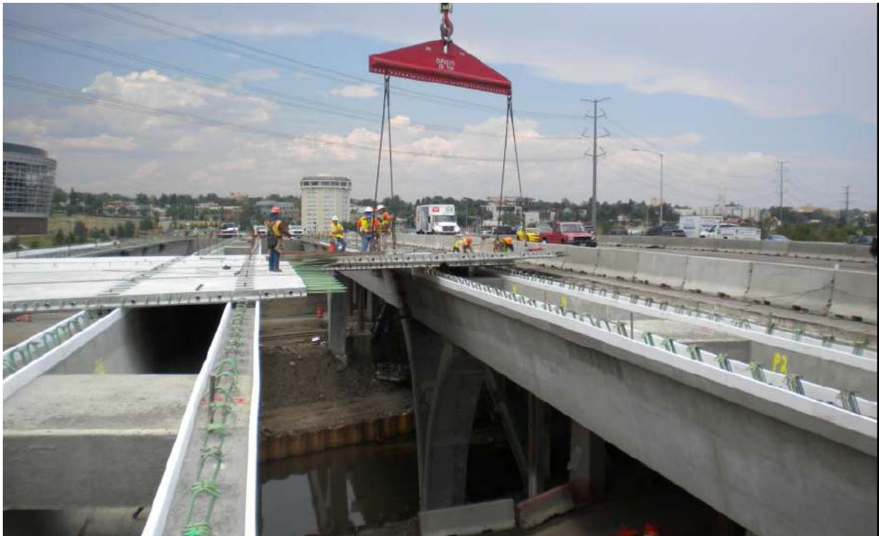
Figure 25. Photo. Panels set with pockets over shear reinforcing in girder top flanges (courtesy: Colorado DOT).
