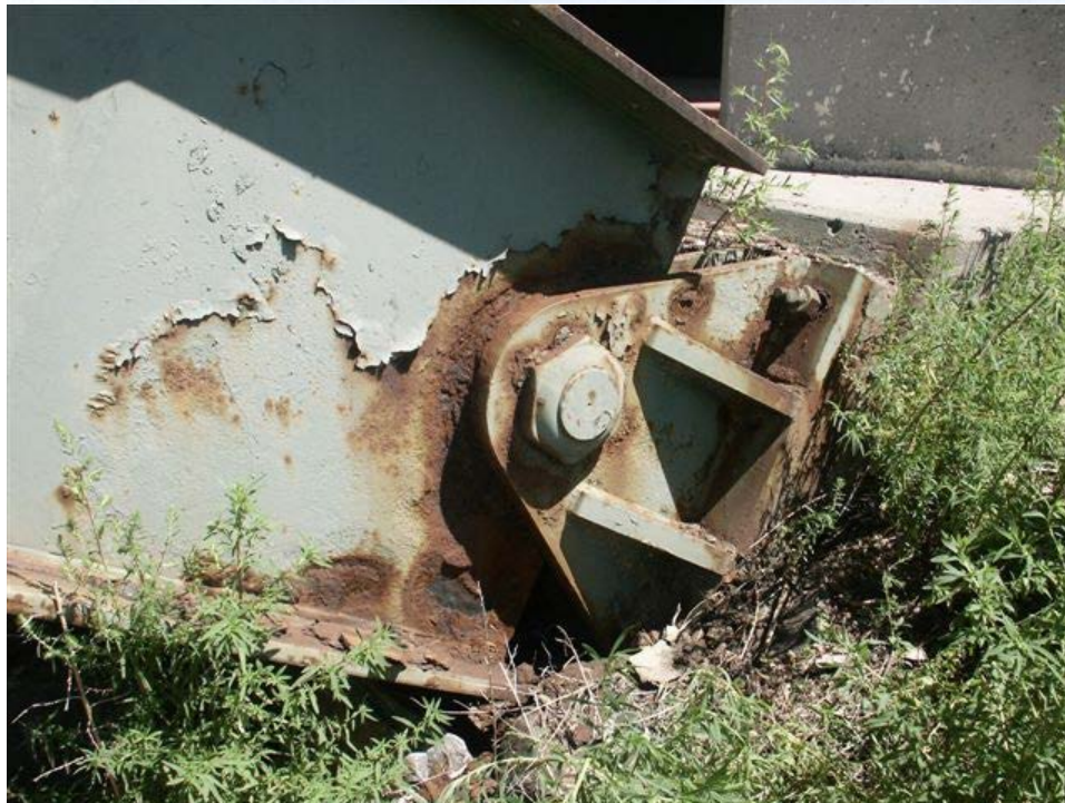
Figure 5. Photos. Deterioration of original structure (courtesy: Colorado DOT).
