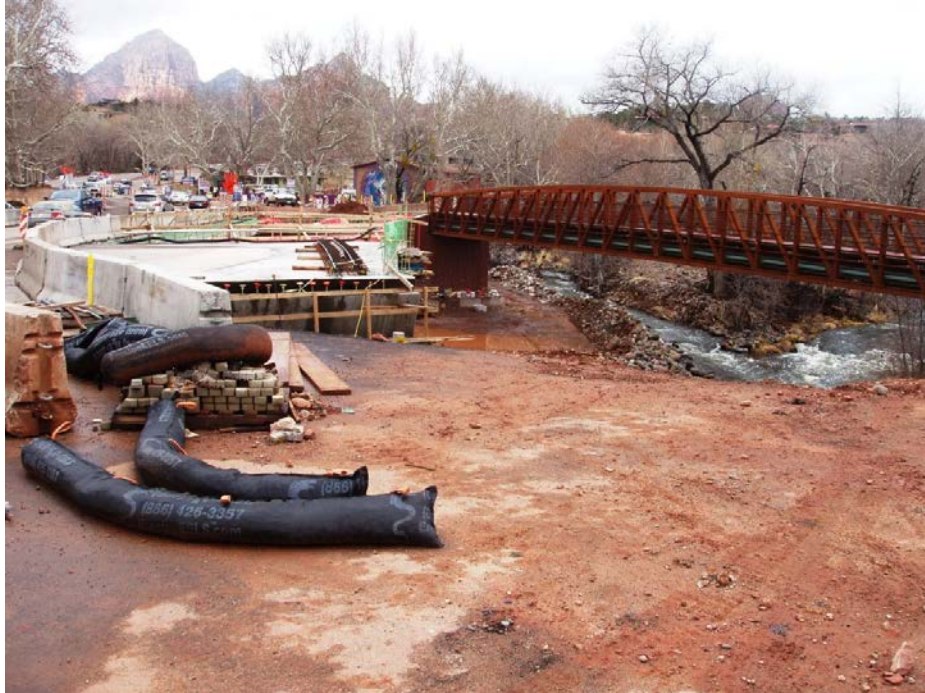
Figure 25. Construction of the first phase of the new Oak Creek Bridge with the already-built pedestrian/utility bridge in the background.
