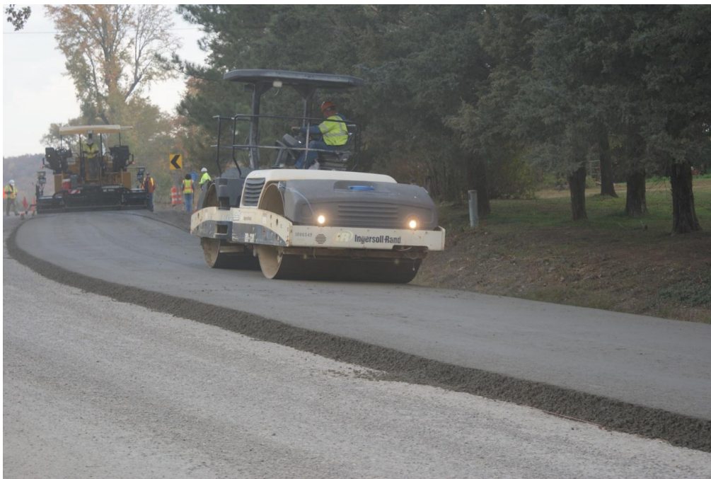
Figure 18. Photo. Larger steel wheel roller (replacing initial light roller) resulting in better compaction and smoother surface.
