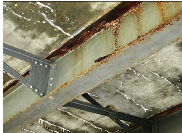
Signs of deterioration in the aging U.S. transportation infrastructure system. (photos: Dr. John J. Myers)
