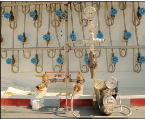
Hydrogen vehicle fueling-station components at Missouri S&T. (photo: Dr. John Sheffield)
