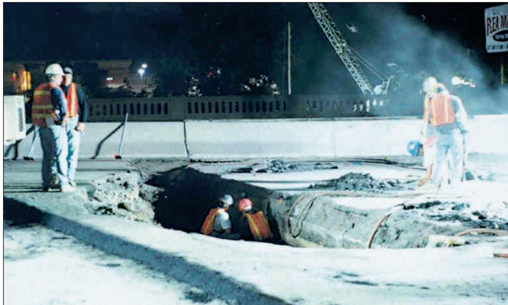
Peckman's River Bridge in New Jersey showing scour damage to approach following Hurricane Floyd. (photo: Dr. M. Ali Khan; from Handbook of Scour Countermeasures Designs Final Report )
