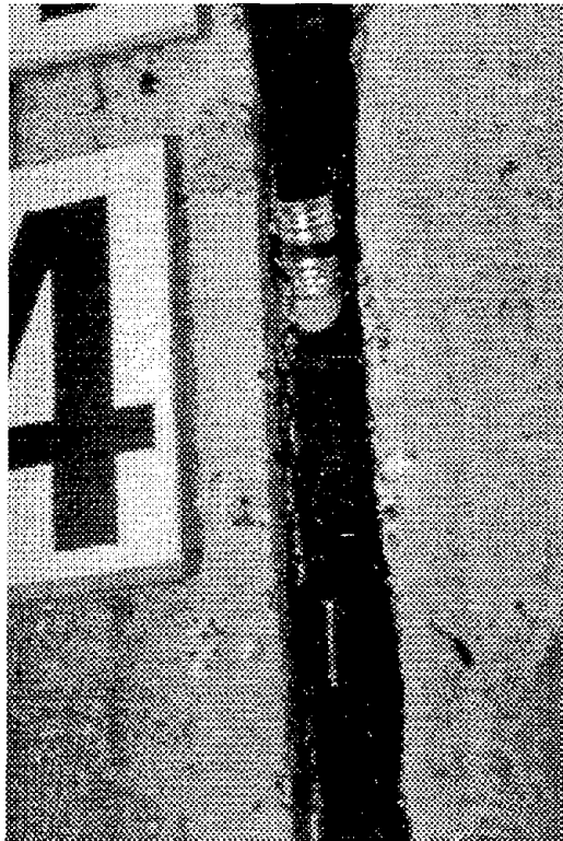
Figure 24. Partial-depth adhesion loss.
