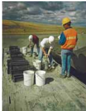
Right: Materials sampling and testing for quality control during construction of the SPS-2 site in Washington State.
