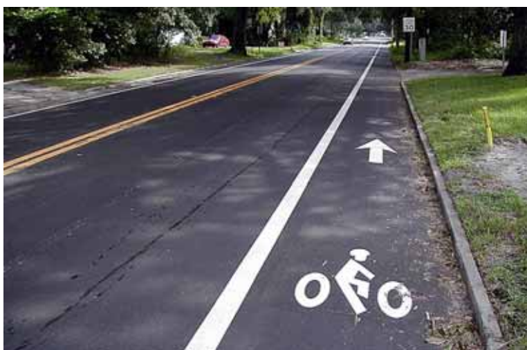
Figure 16-4. Photo. Example of newly striped bicycle lane with accumulation of debris next to curb.
