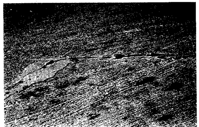
Figure 125. Example of poor sealant application.
