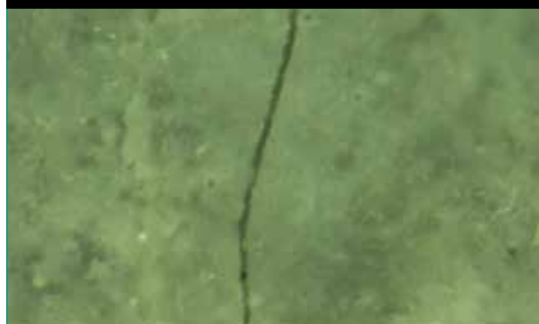
Figure 4. 0.0002-inch (5- \mu m) wide flexural crack in the beam.
