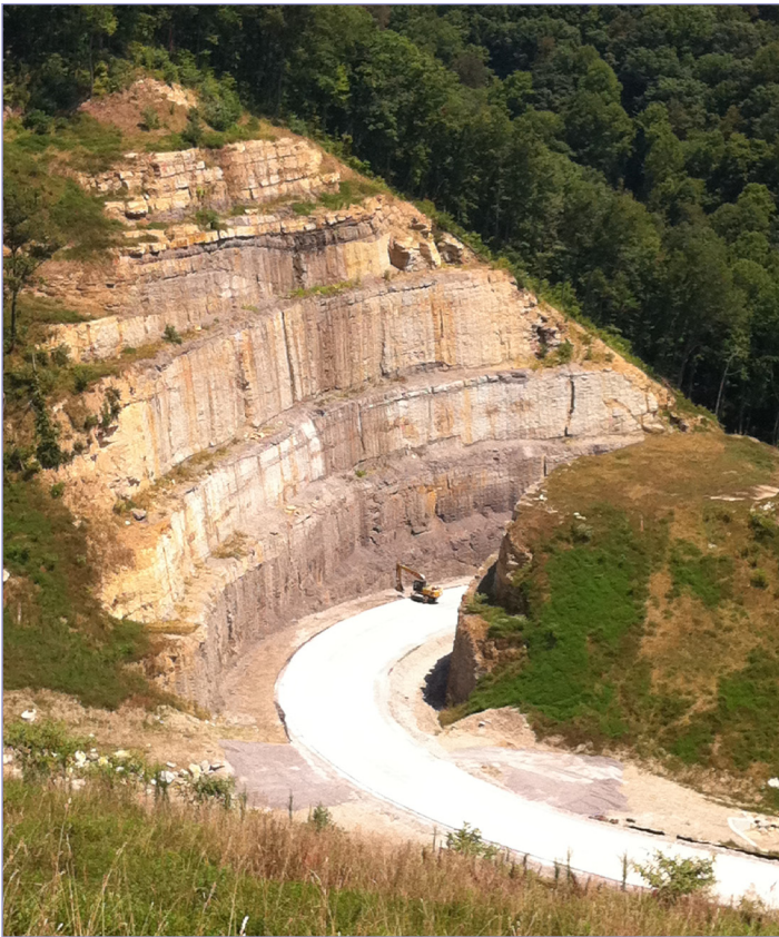
Construction of the I-73/74 NHS Corridor – Red Jacket Section of King Coal Highway
