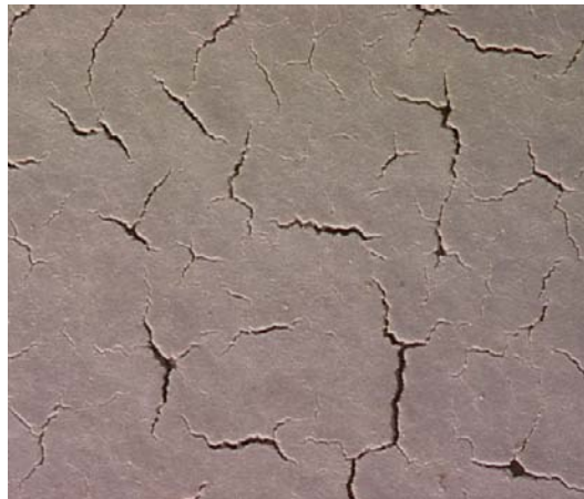
Figure 60. Photo. Surface coating failure by cracking (two-coat system).
