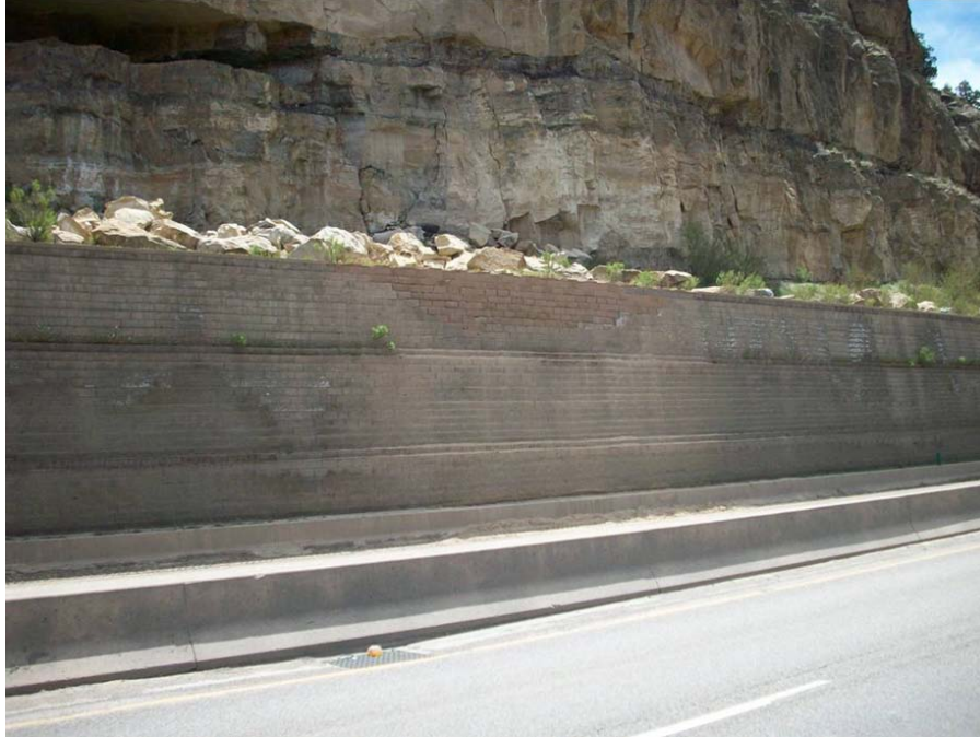
Figure 85. Photo. Repair of a GRS wall after damage caused by rock fall.
