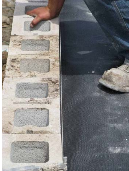
Figure 54. Photo. Checking block alignment with string line reference from back of block.
