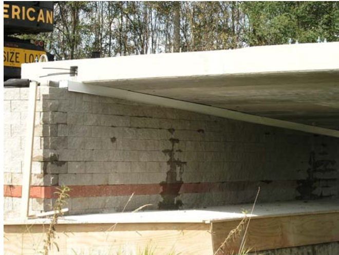
Figure 70. Photo. Aluminum flashing (drip edge) between beams and top of CMU block.
