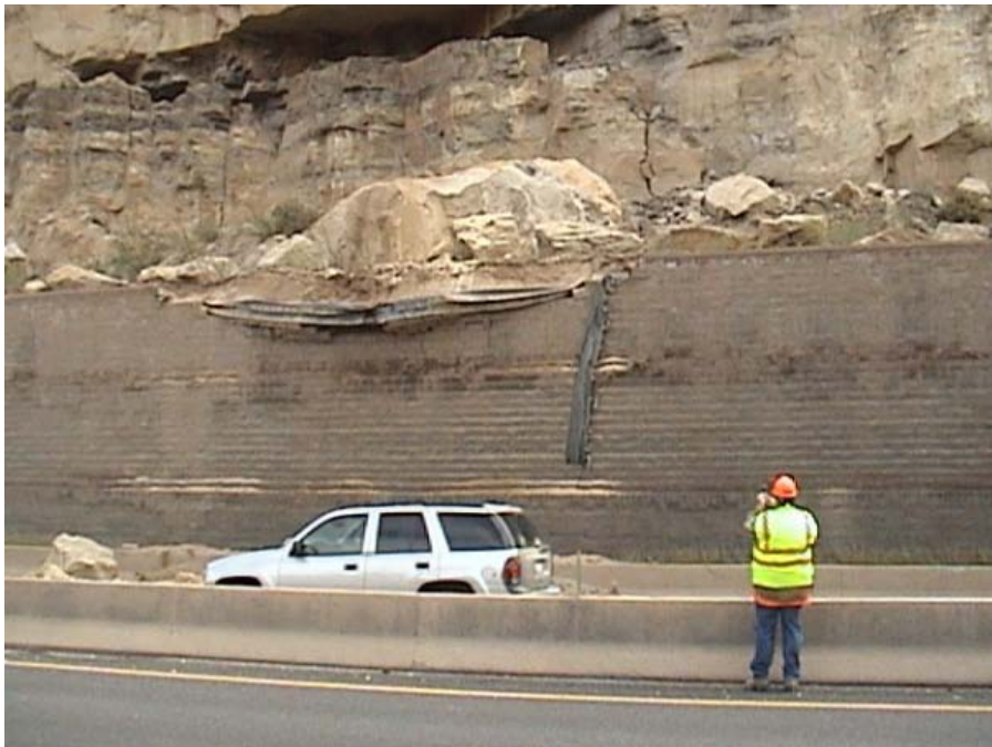
Figure 84. Photo. GRS wall damaged by large sandstone boulder.
