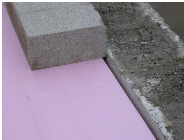
Figure 67. Photo. 4-inch concrete block on top of foam board against top CMU face block.
