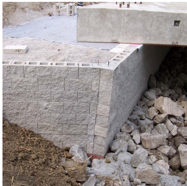
Figure 58. Photo. Vertical seam in wing wall.
