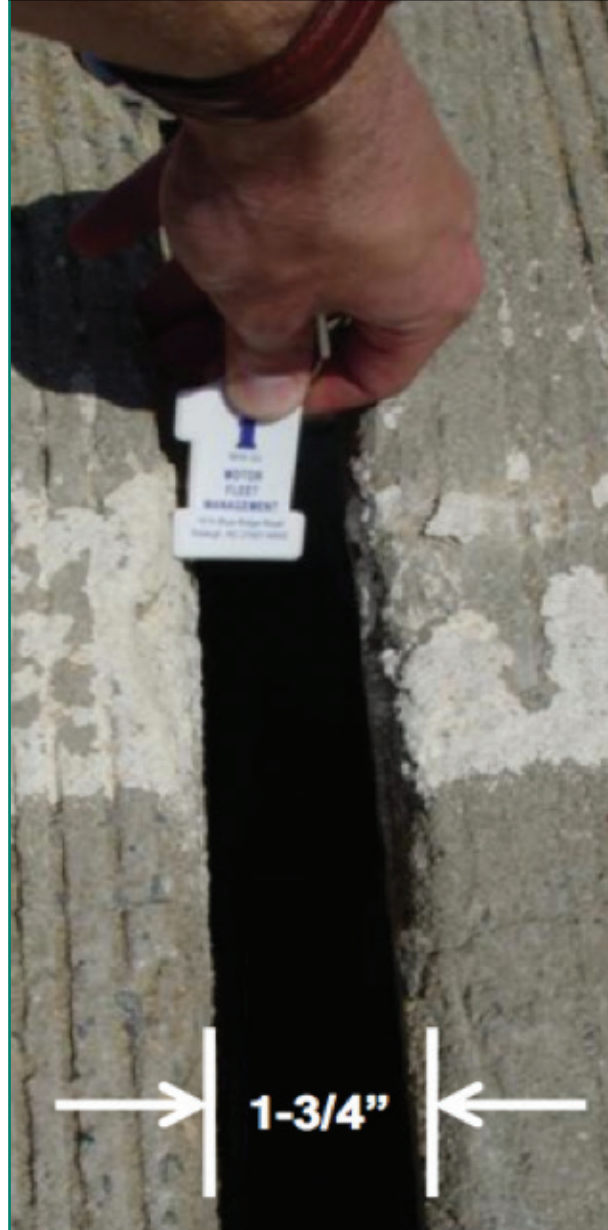
Figure 12. Yadkin River Bridge superstructure distress.
