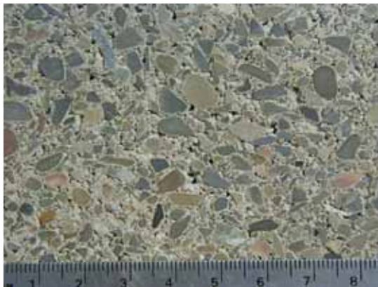
a. SRW mix (note compaction voids).
