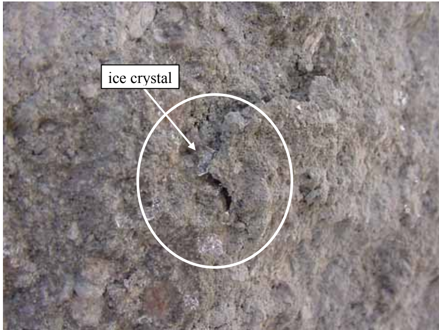
Figure 47. Photo. Breaking off of split face delamination due to ice “jacking” action in field SRW units.
