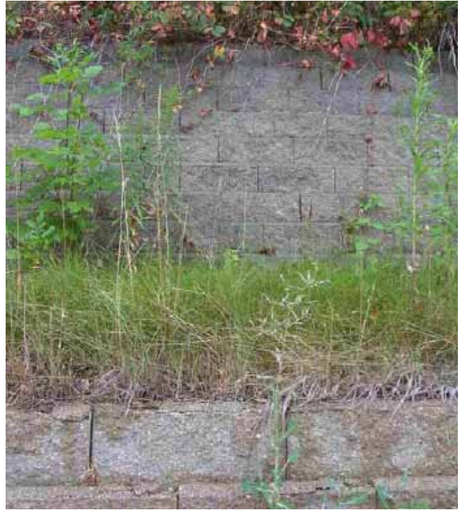
Figure 15. Photo. Deteriorated SRW blocks closest to roadway (bottom of photo) and undamaged SRW blocks farthest from roadway.
