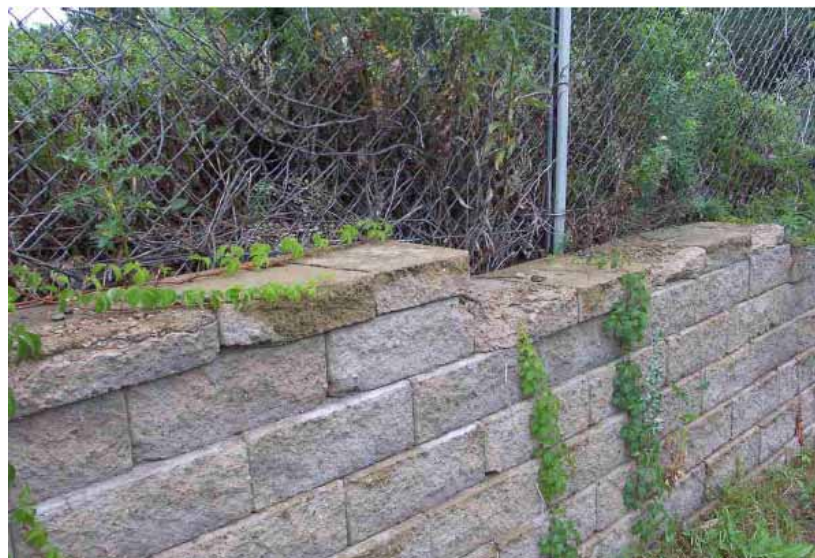
Figure 13. Photo. Severely damaged cap units on otherwise healthy wall.
