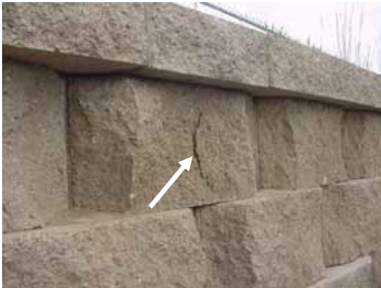
Figure 44. Photo. Sample A of split face delaminations on SRW units.
