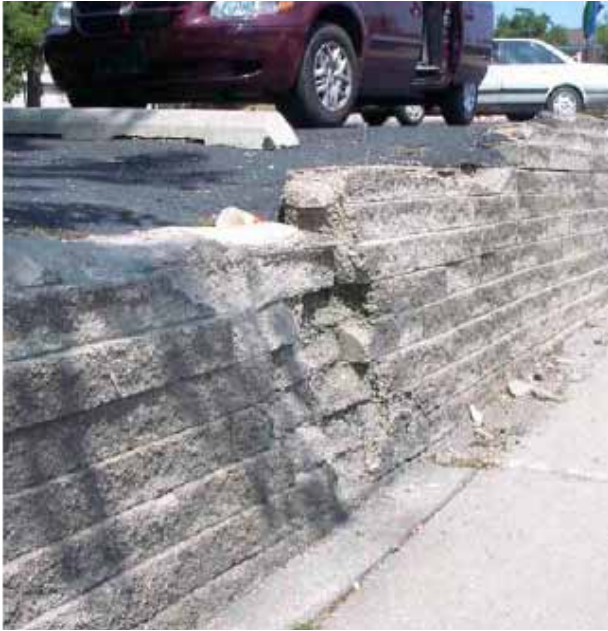
Figure 14. Photo. Effects of drainage and salt exposure from parking lot above SRW.
