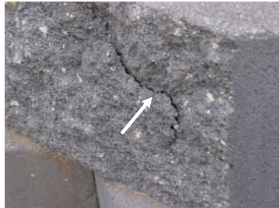
Figure 45. Photo. Sample B of split face delaminations on SRW units.
