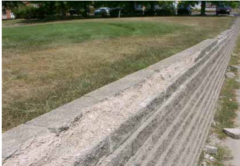
Figure 12. Photo. Typical deterioration of SRW blocks with scaling most pronounced for cap units.
