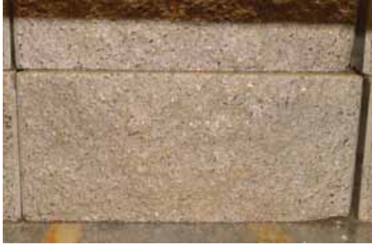
Figure 203. Photo. SHA-approved block from manufacturer A (water exposure).
