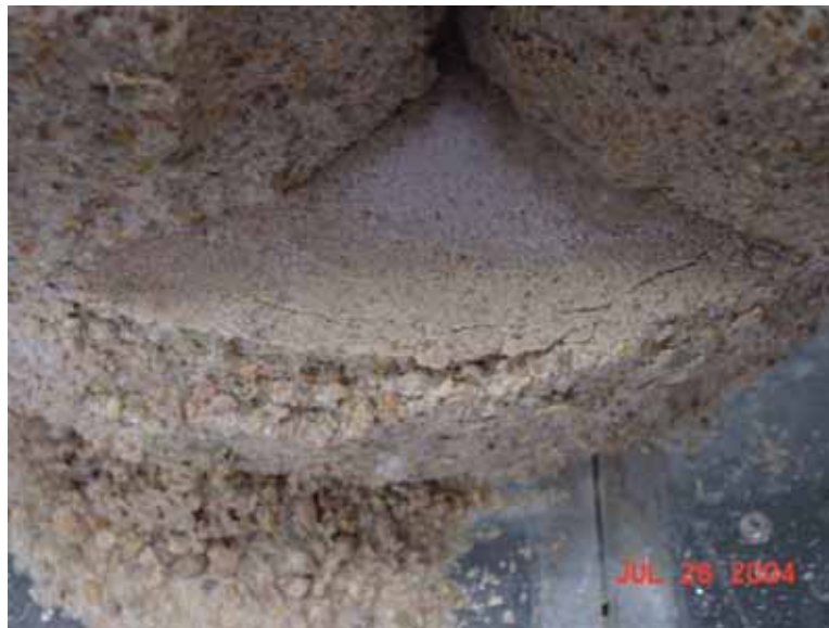
Figure 196. Photo. Typical cracking and spalling from freeze-thaw damage from test 1.
