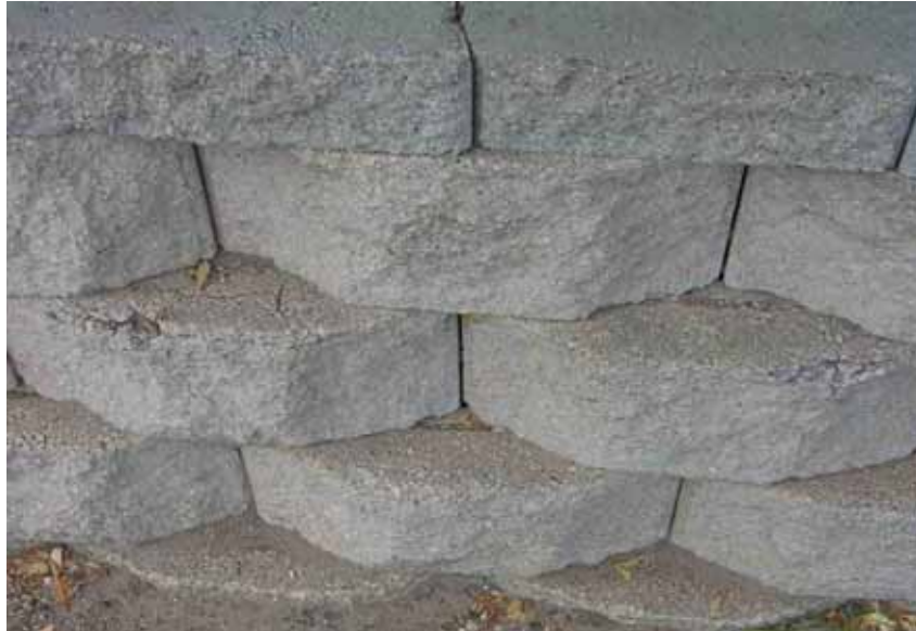
Figure 20. Photo. Another example of deterioration of exposed horizontal surfaces of SRW blocks.
