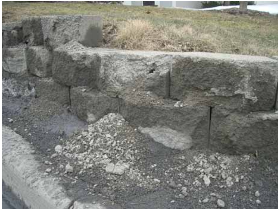
Figure 8. Photo. Condition of SRW in Ithaca, NY.
