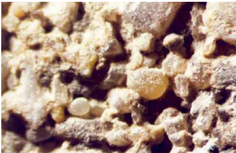
Figure 25. Photo. Internal structure of block from Wisconsin SRW (WI-4), showing large compaction voids and low cement paste content.
