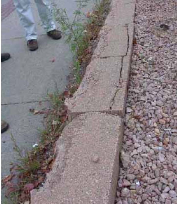
Figure 18. Photo. Cap block experiencing scaling of front face and macrocracking towards the back of the blocks.
