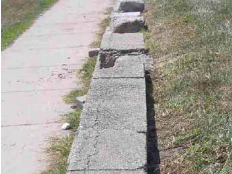
Figure 17. Photo. Deterioration of SRW blocks due to exposure to fertilizers from adjacent golf course.
