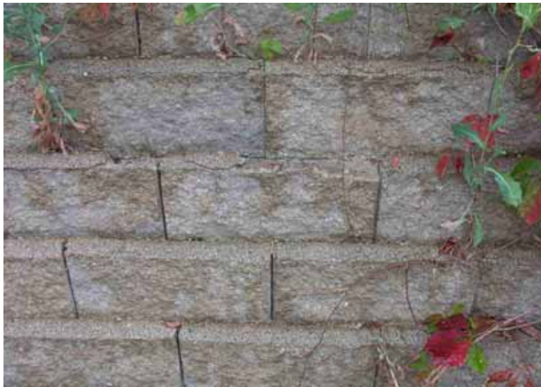
Figure 19. Photo. Deterioration of exposed vertical surfaces of SRW blocks.
