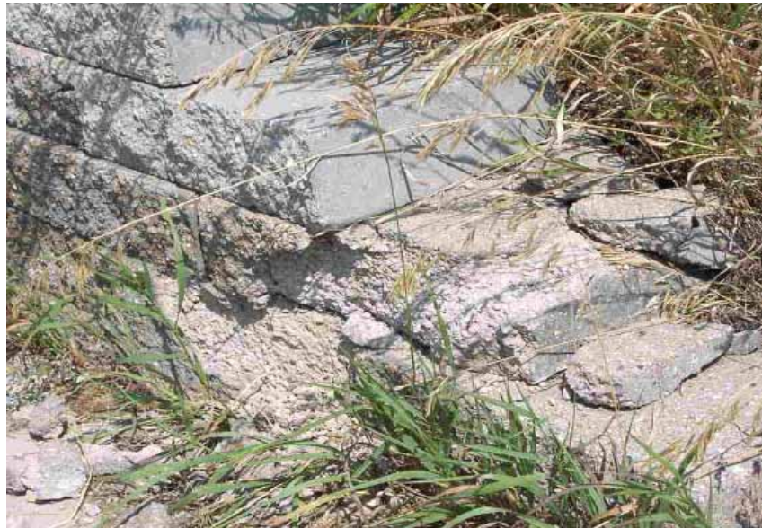
Figure 16. Photo. Severe damage of SRW blocks in direct path of drainage from bridge overpass above.
