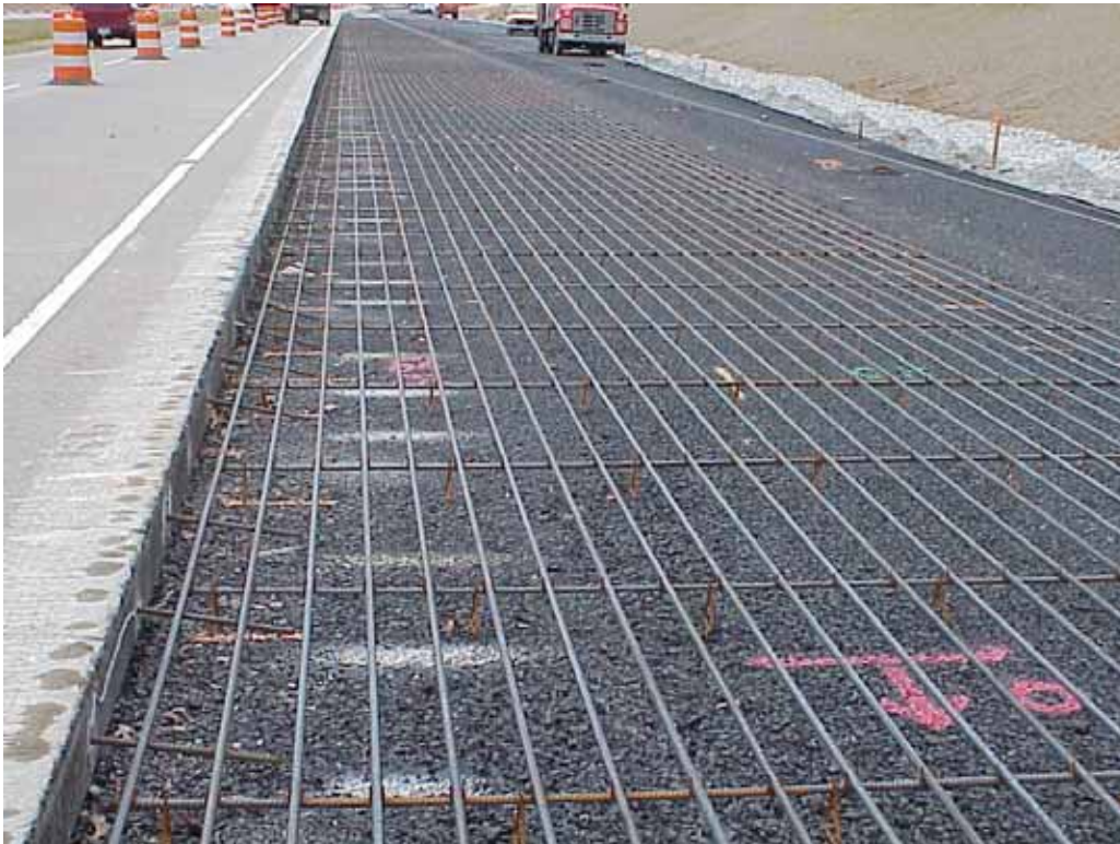
Figure 1. Photo. Typical example of reinforcement layout for CRCP (constructed on S.R. 288 in Virginia). (12)
