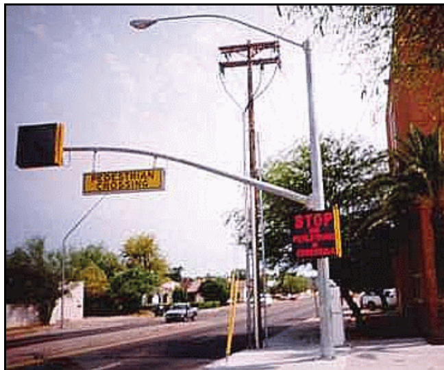
Figure 29. These innovative pedestrian crossing signs had mixed results.
