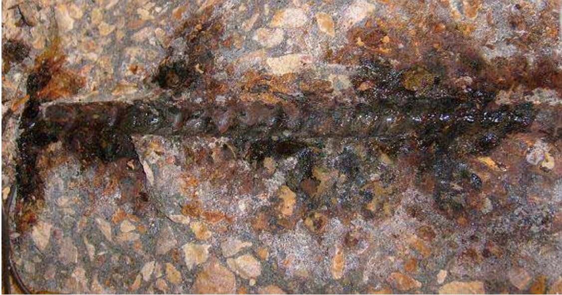
Figure 240. Photo. Top view of specimen Zn-4, 25-mm (1-inch) cover, after autopsy.
