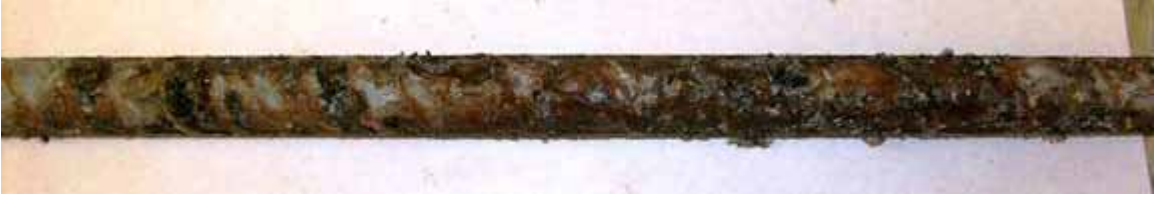
Figure 242. Photo. Top side of galvanized reinforcement, 25-mm (1-inch) cover, after autopsy at crack initiation.
