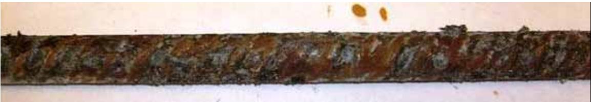
Figure 244. Photo. Bottom side of galvanized reinforcement, 25-mm (1-inch) cover, after autopsy at crack initiation.
