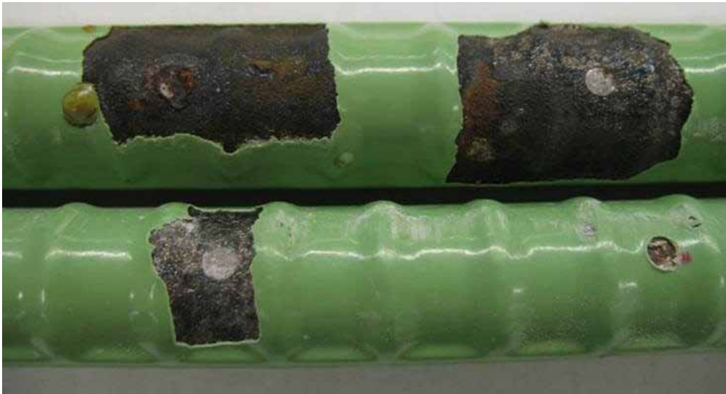
Figure 105. Photo. Conventional epoxy-coated top and bottom bars from southern exposure specimen containing calcium nitrite after 96 weeks.
