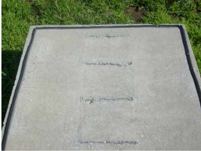
Figure 153. Photo. Field test specimen with simulated cracks containing conventional epoxy-coated steel at 254 weeks.
