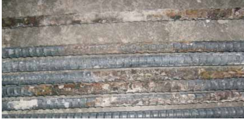
Figure 150. Photo. Top bars from field test specimen without simulated cracks containing conventional reinforcing steel at 254 weeks.
