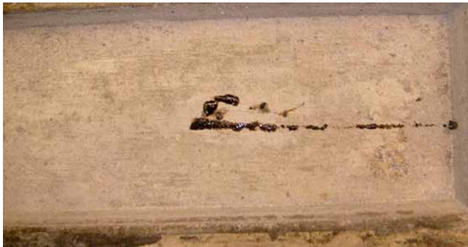
Figure 241. Photo. Staining on surface at crack initiation in galvanized reinforcement specimen, 25-mm (1-inch) cover.
