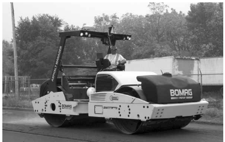
A thin lift of hot-mix asphalt is compacted with an IC roller on U.S. 52 in West Lafayette, IN.
