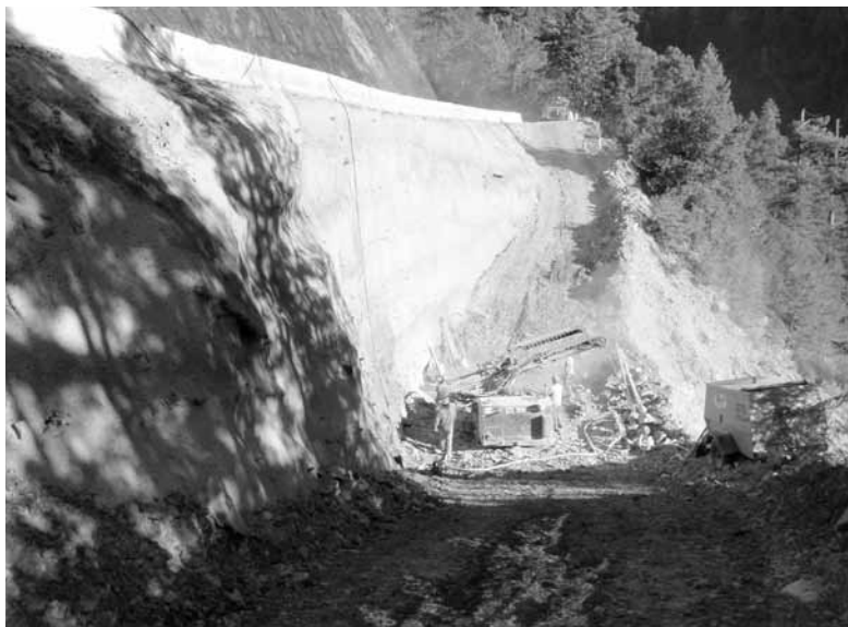
FHWA’s Central Federal Lands Highway Division used hollow bar soil nail technology for a project on South Fork Smith River Road in California.
