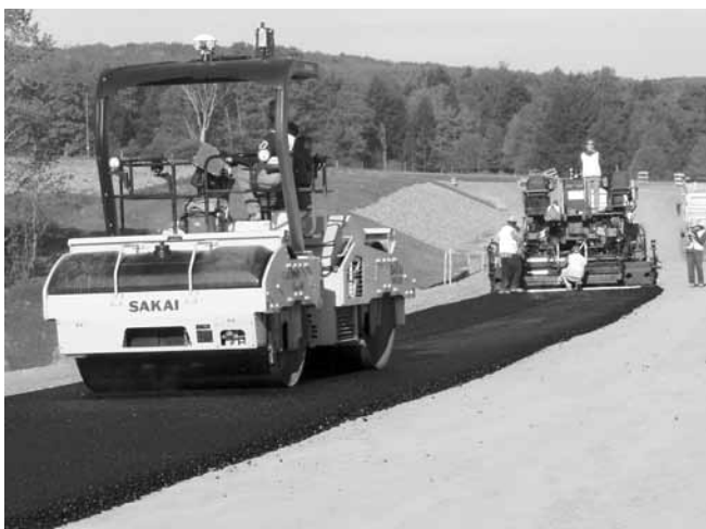
An intelligent compaction (IC) roller is used to place a hot-mix asphalt lift on U.S. 219 in Springville, NY.
