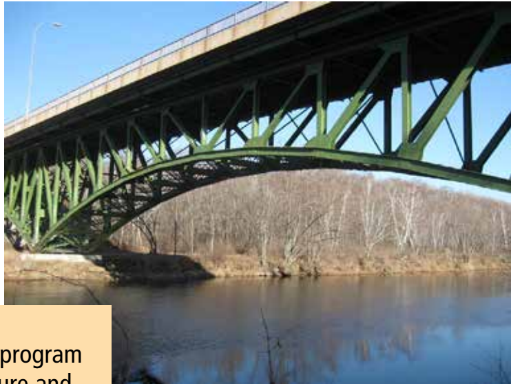
Pilot bridges for the Long-Term Bridge Performance (LTBP) program included this steel deck truss bridge in Sandstone, MN.
