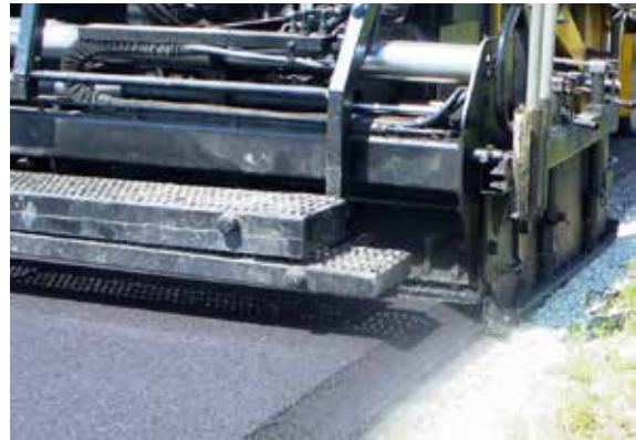
(below) More than 40 States have implemented the Safety Edge SM paving technique, which allows drivers who drift off the roadway to safely and smoothly return to the road.
