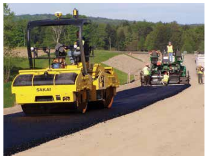
Intelligent compaction rollers accelerate project completion and improve the quality of compaction operations.
