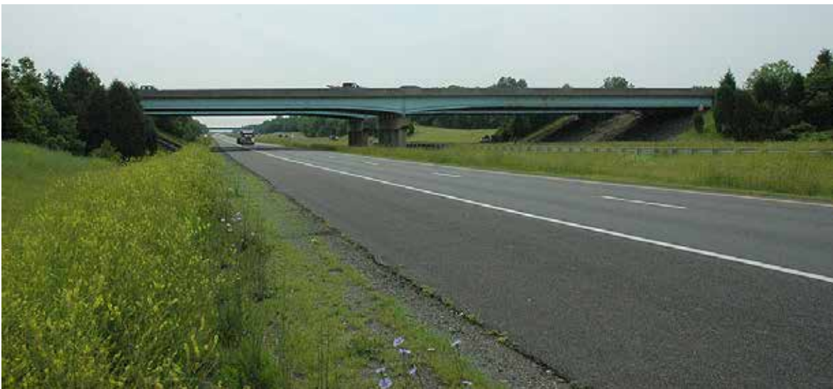
Also studied in the LTBP program's pilot phase was this continuous steel stringer bridge in Prince William County, VA.
