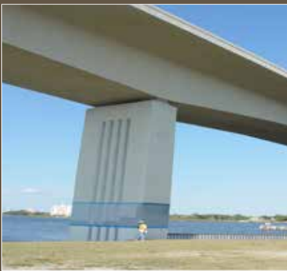
Figure 4. The Florida pilot bridge carries traffic over the Halifax River (Inter-coastal Waterway).
