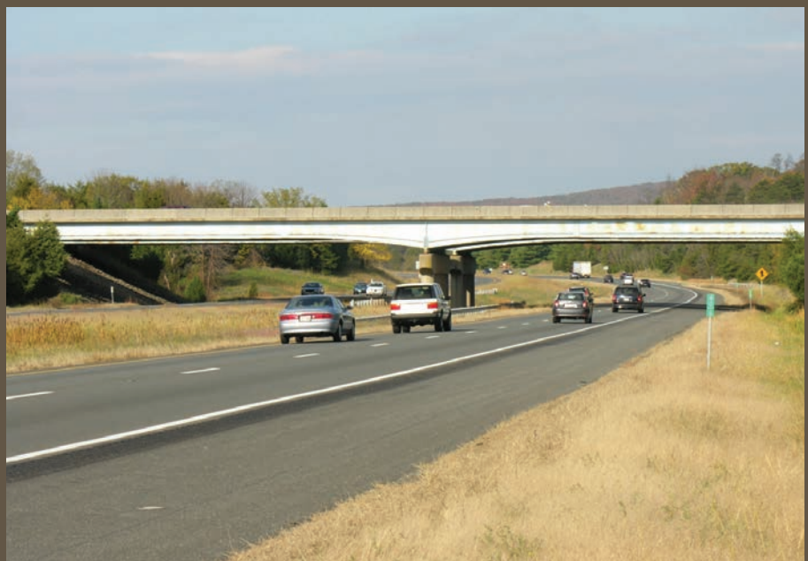
Figure 1. The Virginia Pilot Bridge carrying U.S. Route 15 over Interstate 66 in Haymarket, VA.
