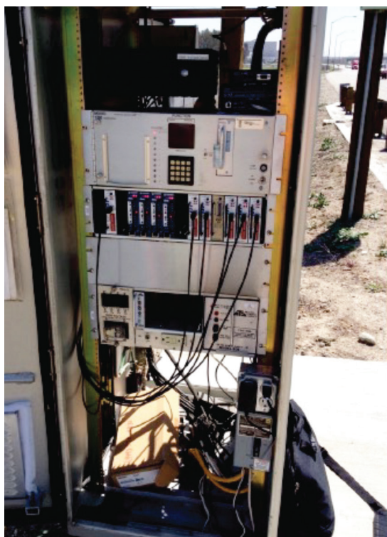
Figure 2. A traffic controller cabinet used to field test a signature-capable detector card.
