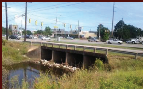
Airport Boulevard Culvert over Montlimar Creek in Mobile, Alabama. Photo credit: Jake Keller (Parsons Brinckerhoff).
