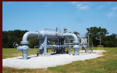
Natural gas pipeline terminal in Mobile, Alabama. Photo credit: Beth Rodehorst (ICF International).
