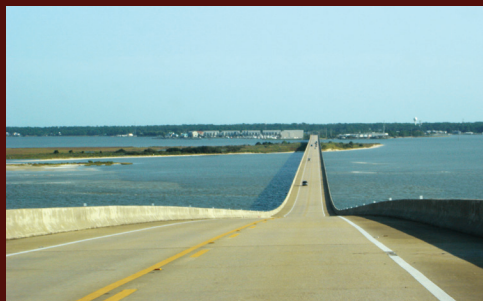
Dauphin Island Bridge in the Central Gulf Coast region. Photo credit: Beth Rodehorst (ICF International).
