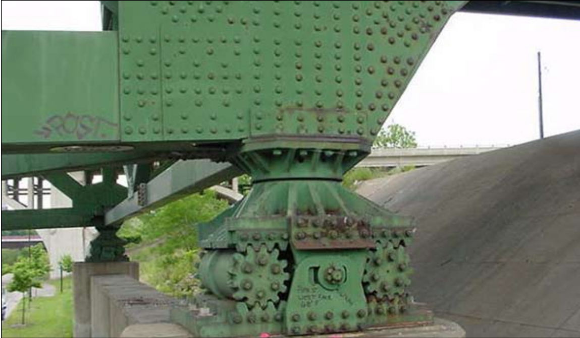
Figure 5. Expansion roller bearings at pier 5, looking east. (Source: URS Corporation)
