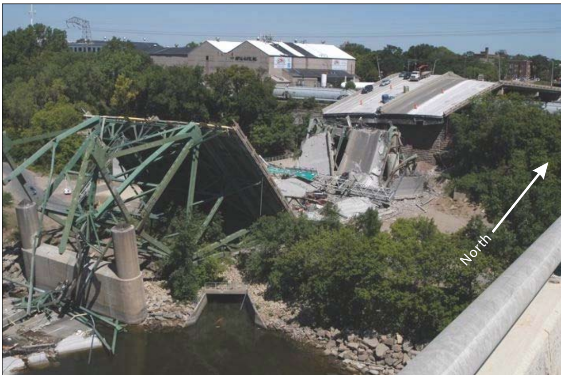
Figure 15. Collapsed north section of bridge.
