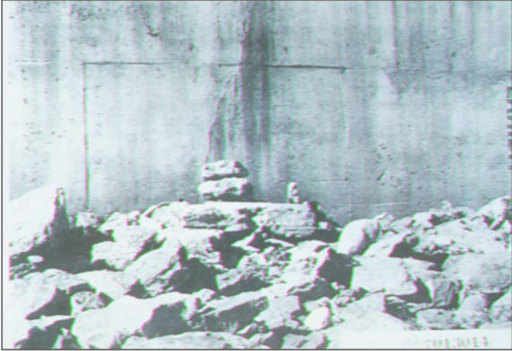
Figure 10.1. Photograph of riprap at pier 2, October 1956.
