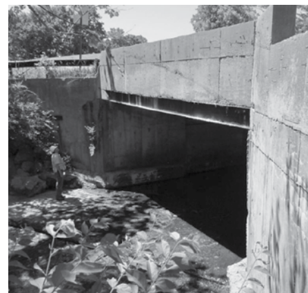
Top: A bridge in North Carolina is inspected using under-bridge inspection vehicles.
