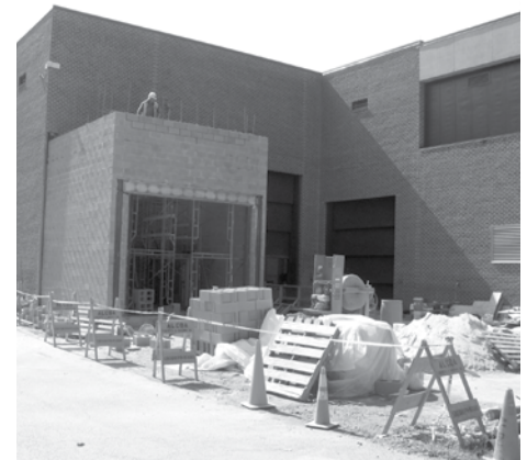
The recent construction of FHWA's expanded Hydraulics Laboratory is enabling major new research studies on bridge scour.
