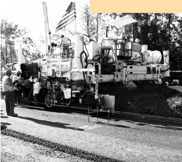
Long-life concrete pavement under construction along a section of I-90 near Syracuse, NY.
