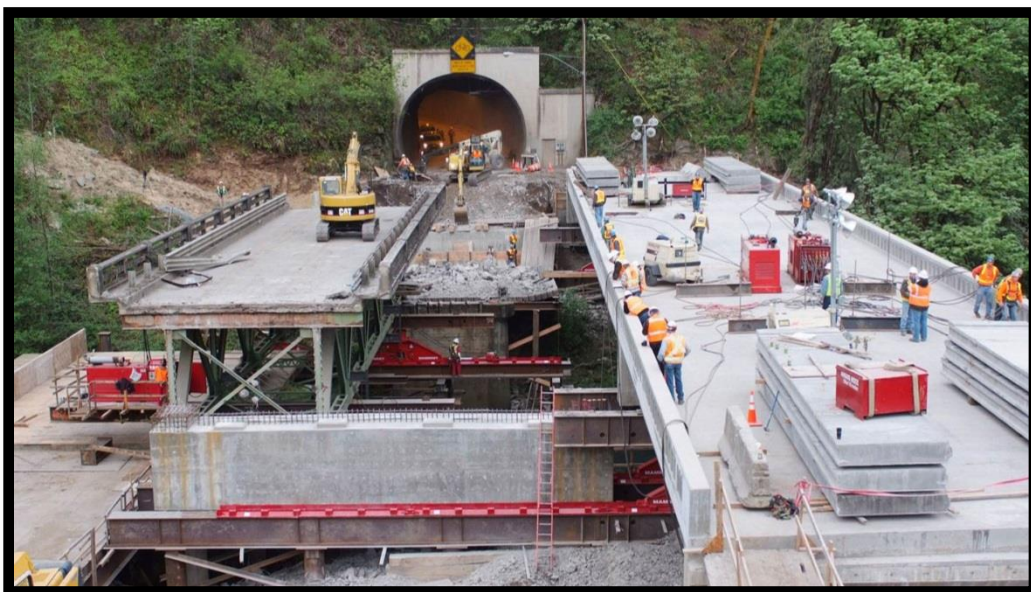
Figure 1-5 SIBC with Constraints Limiting Traffic Control Options at the OR-38 Bridge Project, Oregon
