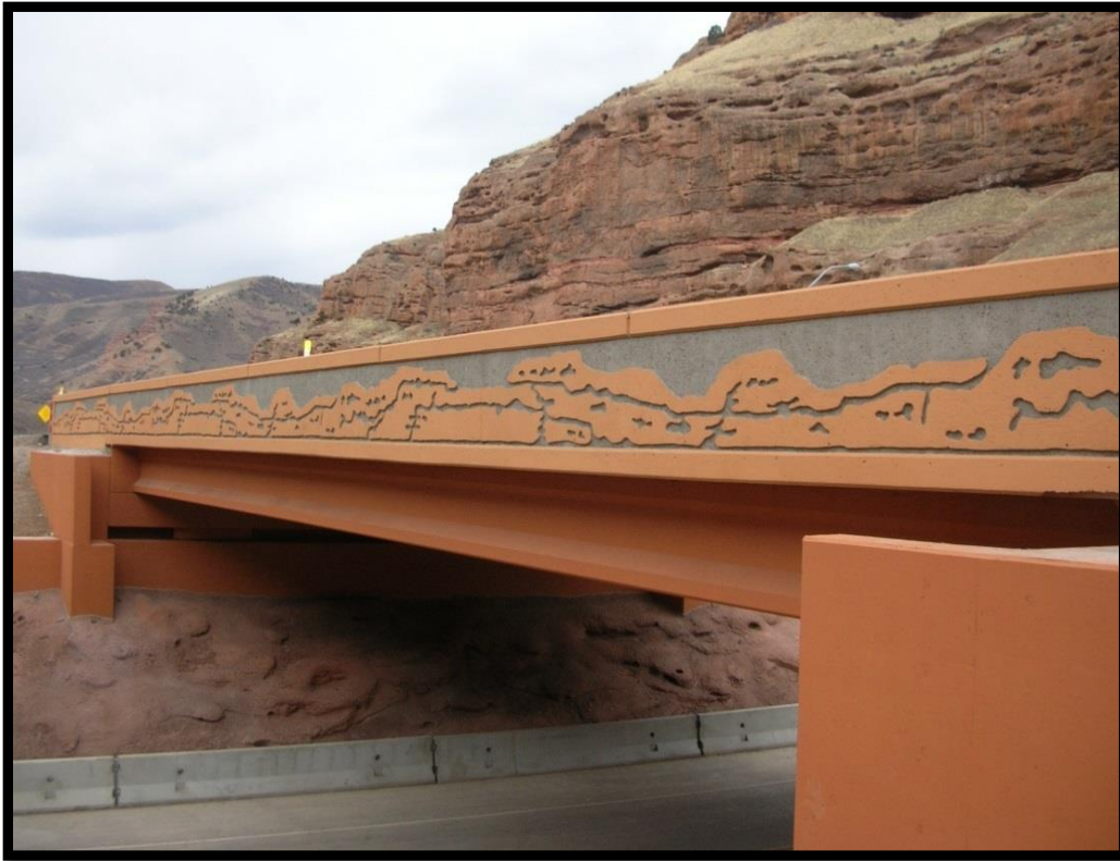
Figure 3-3 Three-Span Overpass Bridge Converted to a Single-Span on the I-80 Echo Road Bridge Project (After)
