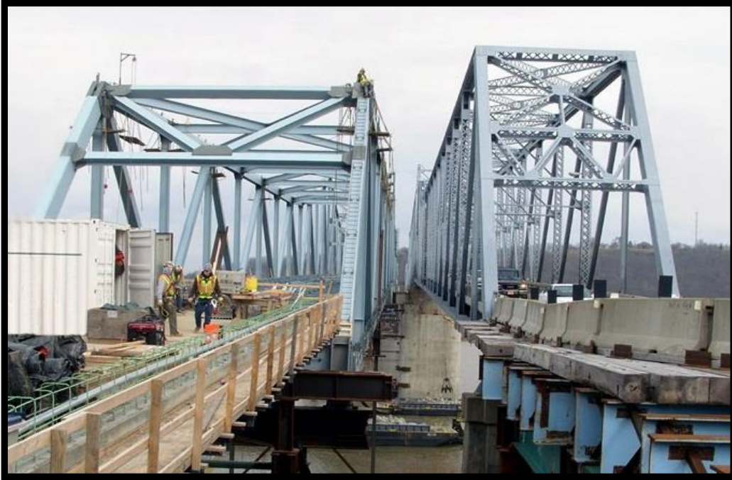
Figure 1-3 SIBC for a Large Truss Bridge on the Milton-Madison Bridge Project, Indiana/Kentucky
