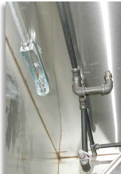
This mock-up hood system plenum space shows the typical placement of fire extinguishing system equipment.
