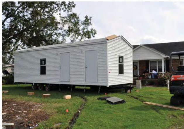
FEMA contractors placing a temporary housing unit on the private site. Source: FEMA
