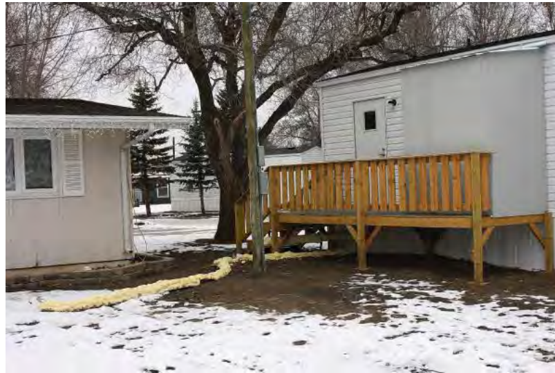
A winterized unit installed on a private site in North Dakota. An arctic room was constructed, insulated skirting was added, and spray foam was also added to insulate the utility lines. Source: FEMA
