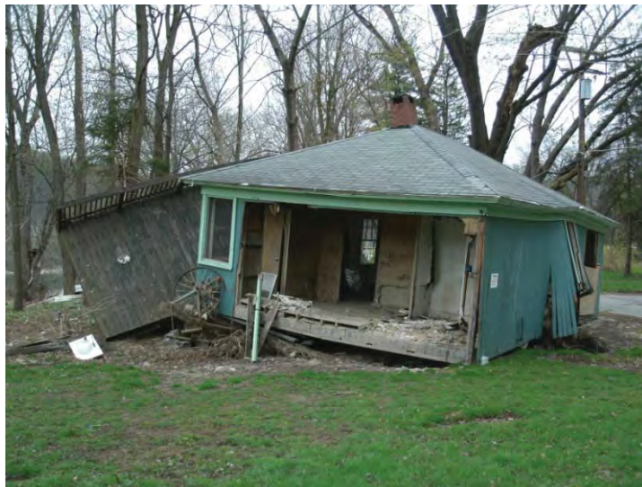
Flood-damaged home in Pennsylvania. Source: OIG
