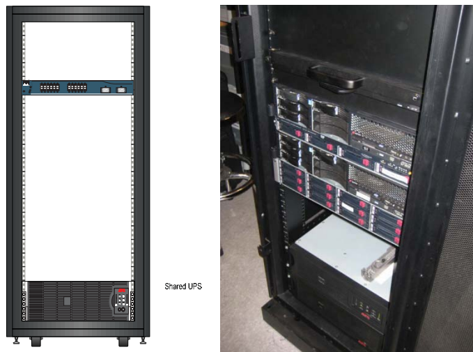
Figure 3: TSA rack diagram from internal TSA report (left) and picture of the same TSA cabinet onsite (right).
