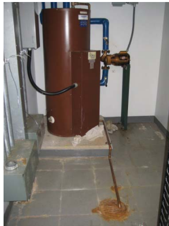
Figure 1: Water heater in room with CBP telecommunications rack.
