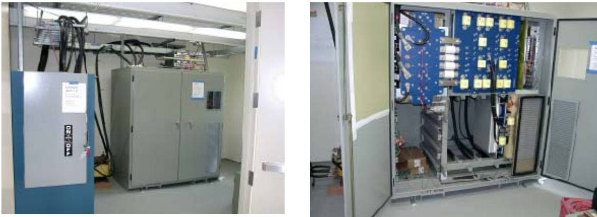
Figure 5. DC rectifier (left) and inverter (right)
