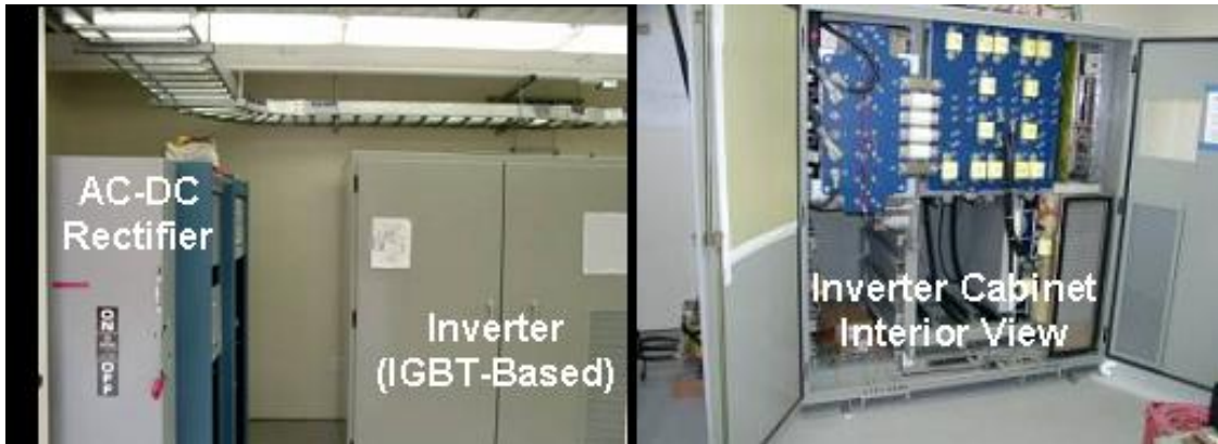
Figure 1-8 View of electrical room, which houses the rectifiers, variable frequency inverter, and train protection equipment
