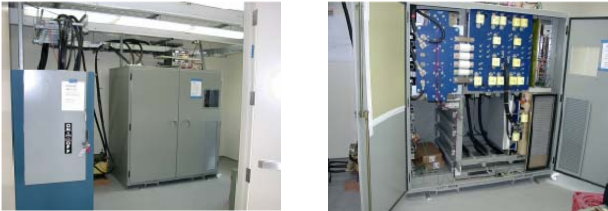
Figure 3.3-6 DC rectifier (left) and inverter (right)
