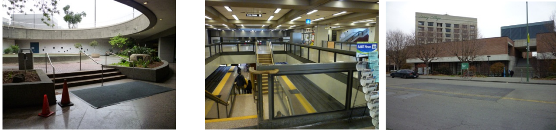
Figures from left-right: Lake Merritt station looking towards fountain, Lake Merritt station looking down to tracks, large exposed vent grate in Madison Ave.
