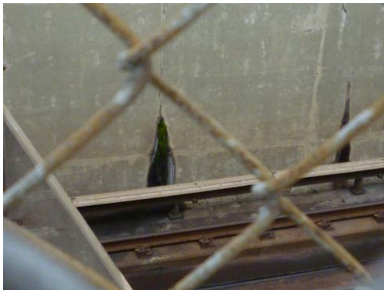
Figure 3-9 Water Damage at Oakland West Portal
