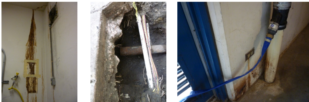
Figures from left-right: Leak stains in Fruitvale train control room, end of down pipe outside of train control room, temporary connection inside of train control room from down pipe to outside walkway.
