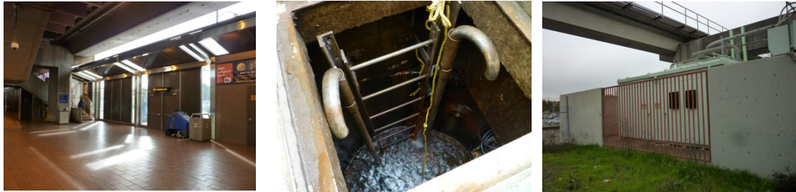
Figures from left-right: Open area between station walls and roof at Oakland Coliseum, pump sump at underpass, train control room.
