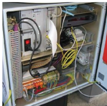
Centralized processing equipment.
