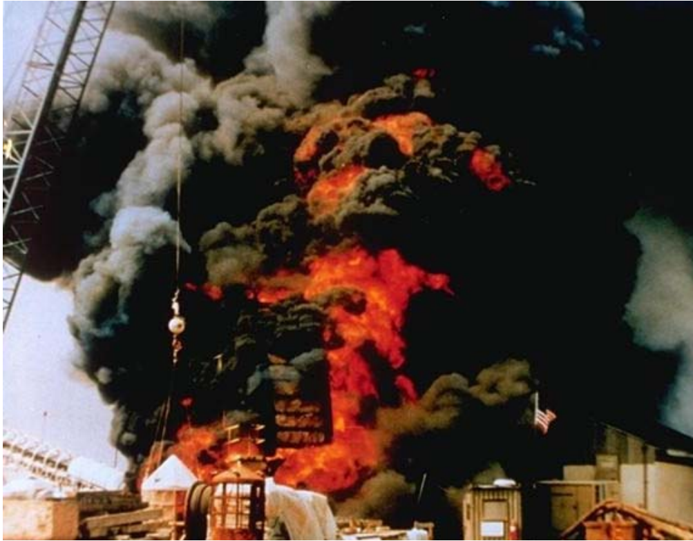
Figure 14-6 Fire in Work Shaft
