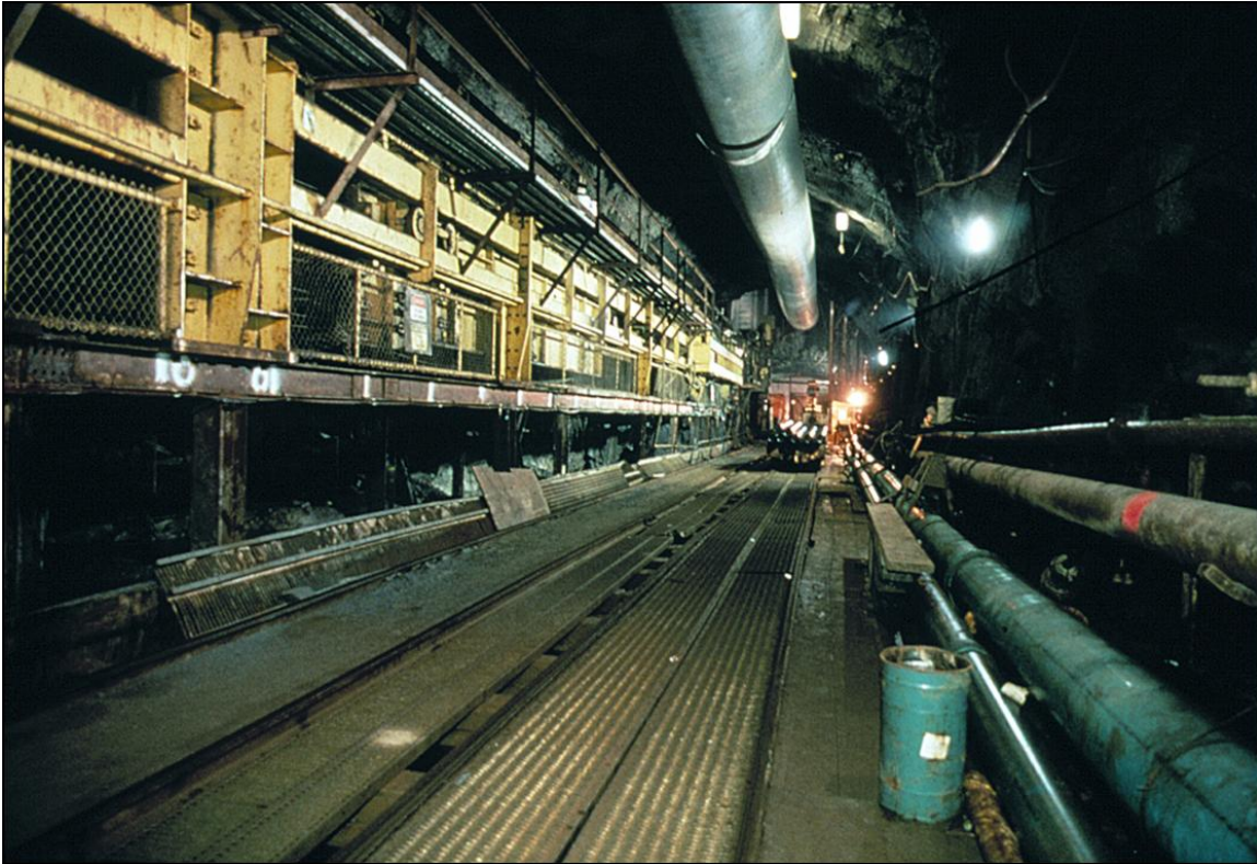
Figure 14-3 Horizontal Muck Conveyor
