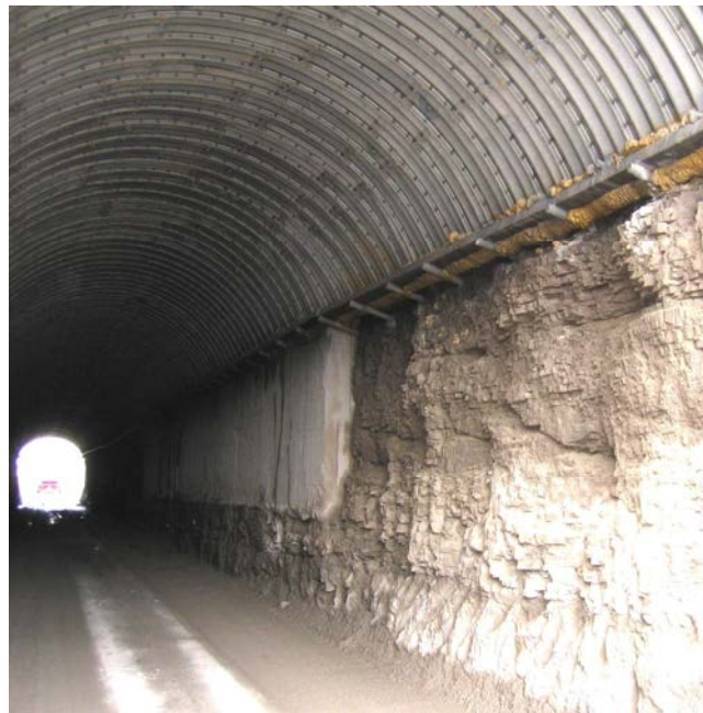
Figure 16-19 Rock Tunnel with Shotcrete Wall Repair and Arch Liner (I-75 Lima Ohio)
