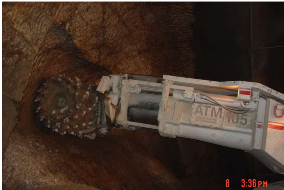
Figure 9-12 Road Header SEM Excavation in Medium Hard, Jointed Rock (Devil's Slide Tunnels, California)
