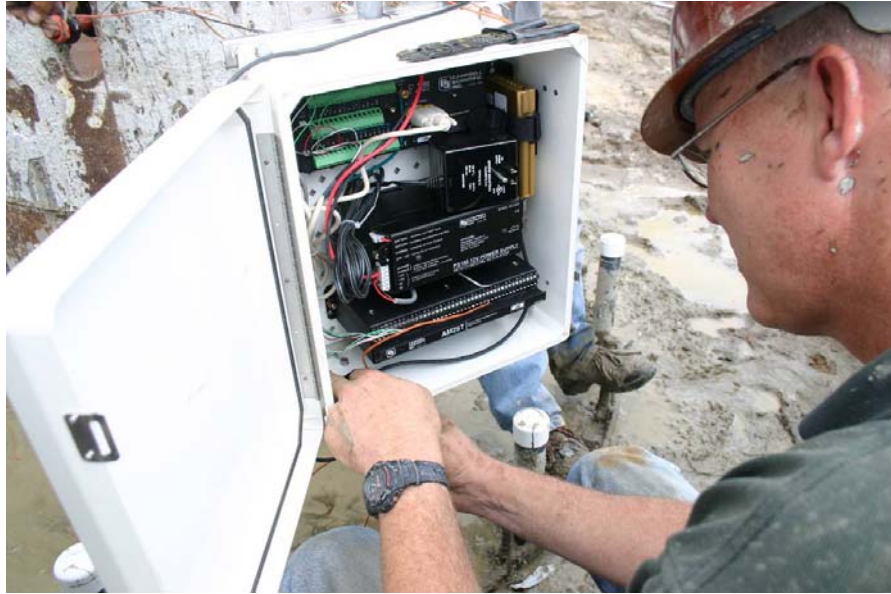
Figure 39. Photo. TC wire connection from AM25t 25-channel multiplexer to CR1000 data logger.
