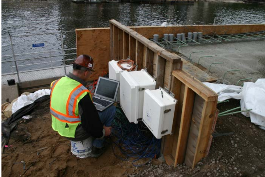
Figure 97. Photo. Temporary DAS system reconnected, reconfigured, and reattached in new location adjacent to the permanent DAS subpanel vault.
