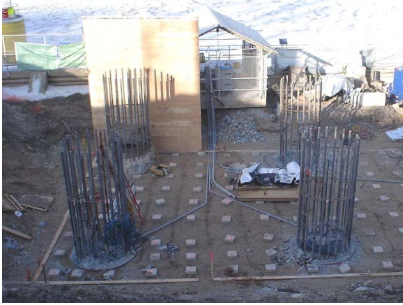
Figure 52. Photo. Conduits running from shafts to DAS boxes.
