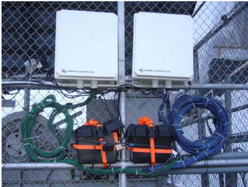
Figure 76. Photo. Construction load monitoring systems (VW = blue (right) and RT = green (left)).
