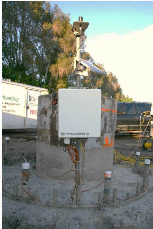
Figure 40. Photo. Remote thermal monitoring system for voided shaft.
