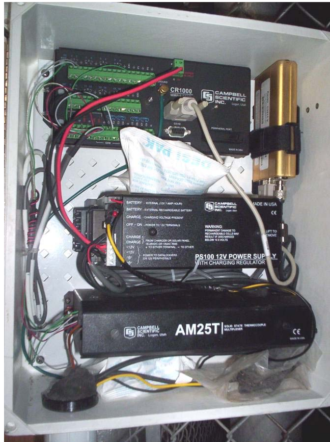
Figure 55. Photo. Thermal monitoring DAS for I-35W bridge shafts.
