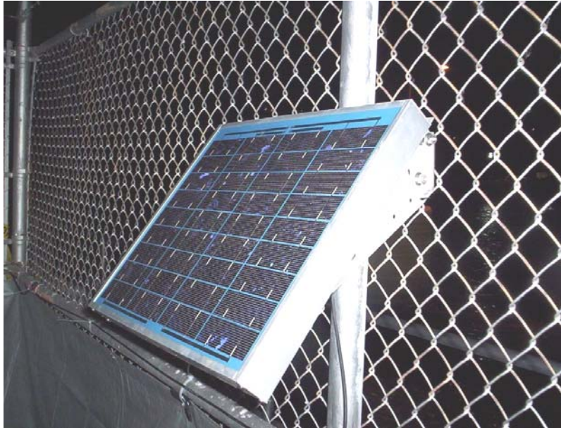
Figure 56. Photo. 35-W solar cell panel for I-35W bridge monitoring system.
