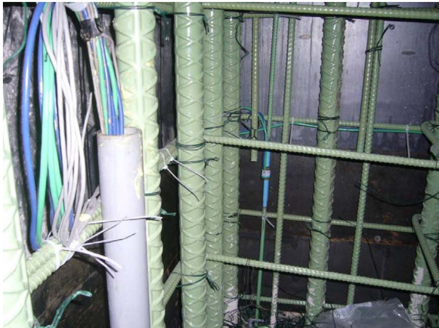
Figure 74. Photo. Wires exiting through conduit.
