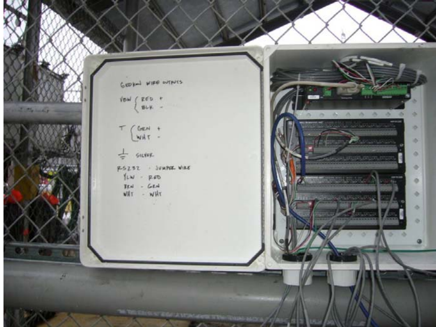
Figure 75. Photo. Wire connection to system 2.
