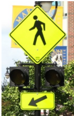
Figure 81. Photo. Circular beacons used at MK-05.
