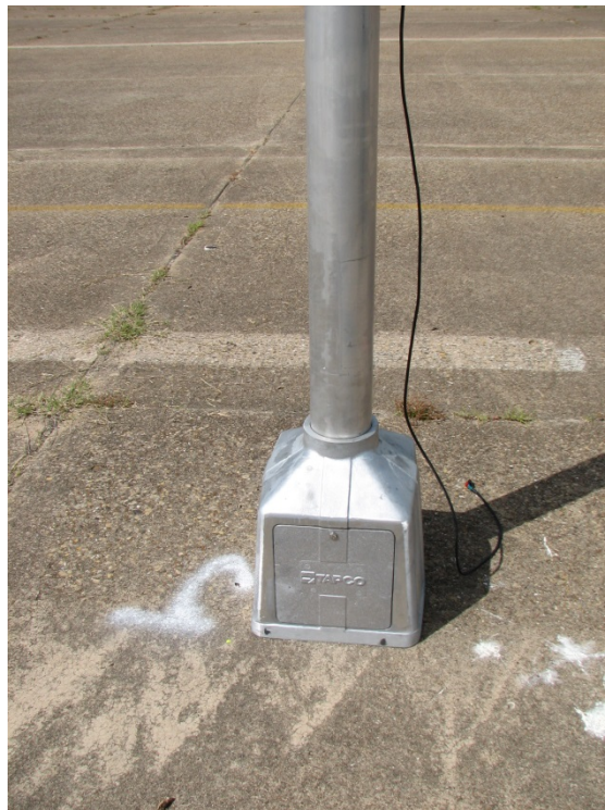
Figure 54. Photo. Base for signs with beacons/LEDs.
