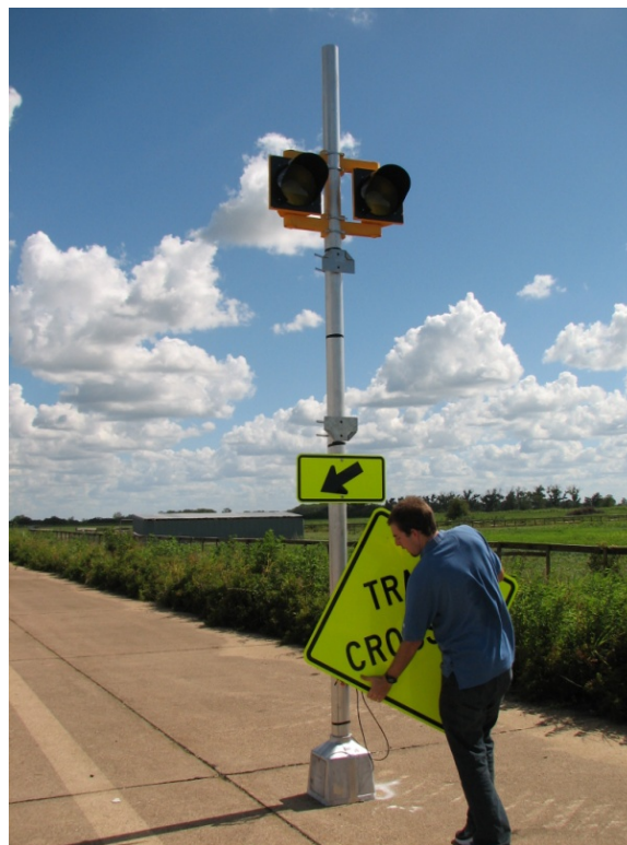
Figure 55. Photo. Example of sign change.
