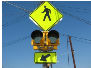
Figure 78. Photo. Circular beacons used at AU-01.
