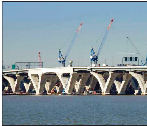
The Woodrow Wilson Bridge is a major project in the Washington, DC, metropolitan area.
