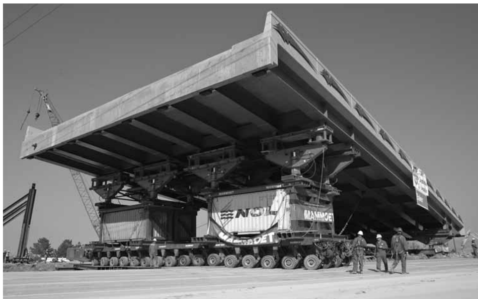
The Utah Department of Transportation used self-propelled modular transporters (SPMTs) to install the prefabricated superstructure of the 4500 South bridge in Salt Lake City in October 2007.
