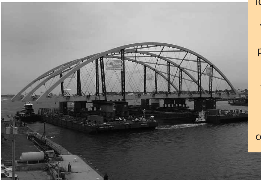
The superstructure for Rhode Island's Providence River bridge was prefabricated a dozen miles away and transported using two barges to the bridge site in August 2006, accelerating the construction process.
