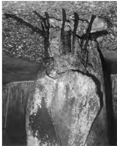
Figure 10-1 Damage to the head of battered piles at the Port of Oakland (after Serventi, 2004)
