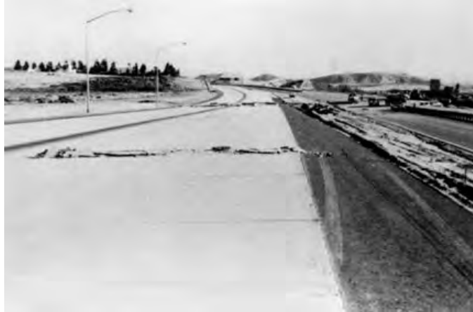
Figure 7-11 Rigid pavement on I-5 south of I-5/I-210 interchange that sheared and buckled at two localities during the 1971 San Fernando earthquake due to 6.5 ft (2 m) of lateral spread displacement.
