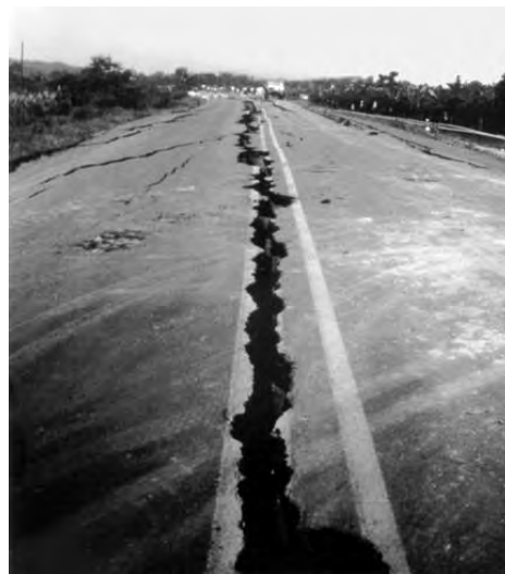
Figure 7-9 Segment of Highway 36 Near Caribbean Coast in Costa Rica that Split Longitudinally, Settled and Spread Laterally during 1991 Earthquake by Mechanism
