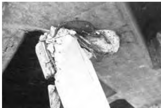
Figure 1-11 Shear Failure of the Head of a Pile at the Struve Slough Bridge
