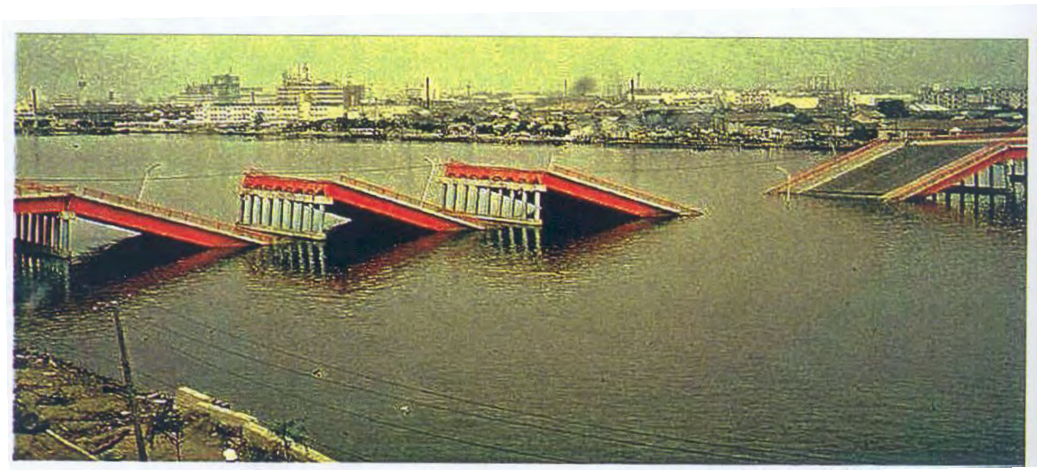
Figure 7-15 Showa Bridge Collapse (Hamada, 1992)
