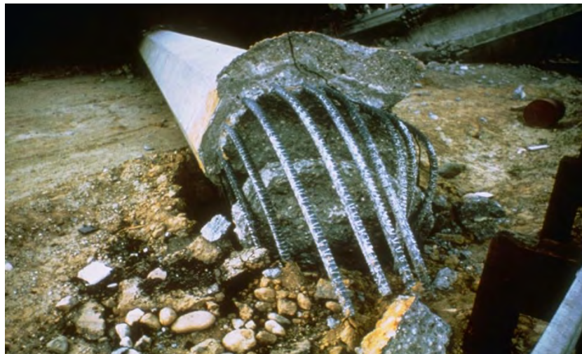
Figure 1-14 Failure of a Bridge Column – Foundation Connection
