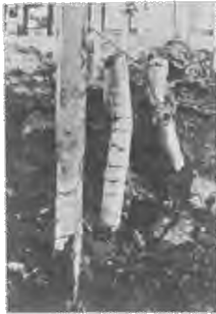
Damage to Foundation Piles of the Hotel Niigata Building
