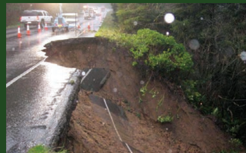
Road collapse along U.S. 101 after extreme storms. Photo credit: Oregon Department of Transportation
