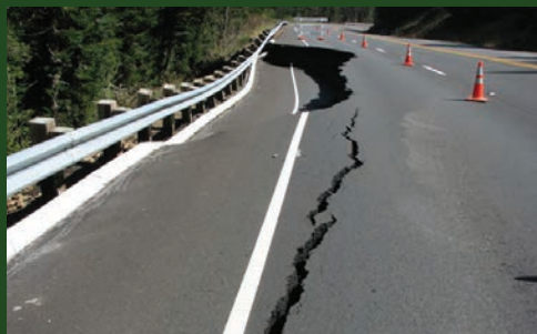
A failed section of U.S. 101 after extreme storms in March 2012. Photo credit: Oregon Department of Transportation
