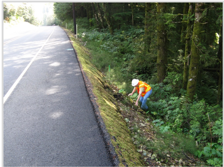
A member of ODOT's project team scrambles up the steep fill slope at Falcon Cove.
