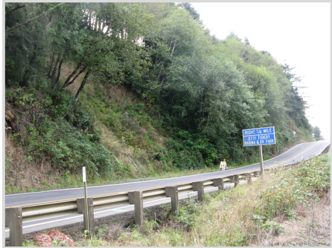
This active section of the Jetty Creek landslide is deforming U.S. 101.
