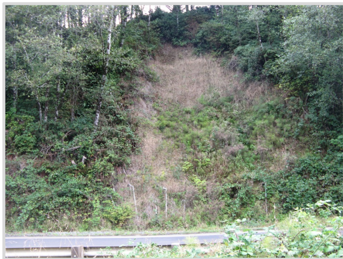
ODOT crews have installed horizontal drains in this section of the Jetty Creek landslide.
