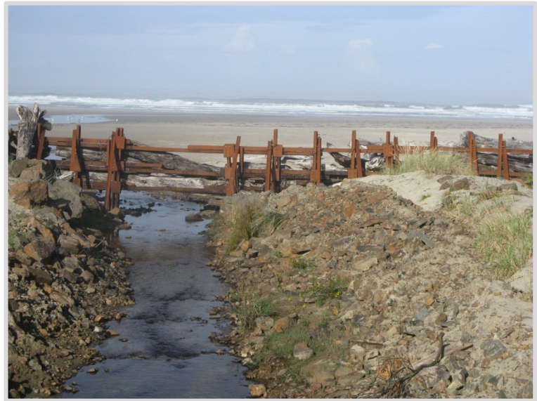
The debris rack at the Salt Air Creek beach outfall.
