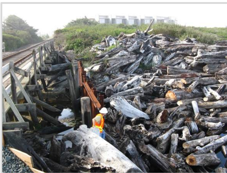
A logjam of driftwood collects in the debris rack at the Crescent Creek outfall adjacent U.S. 101.
