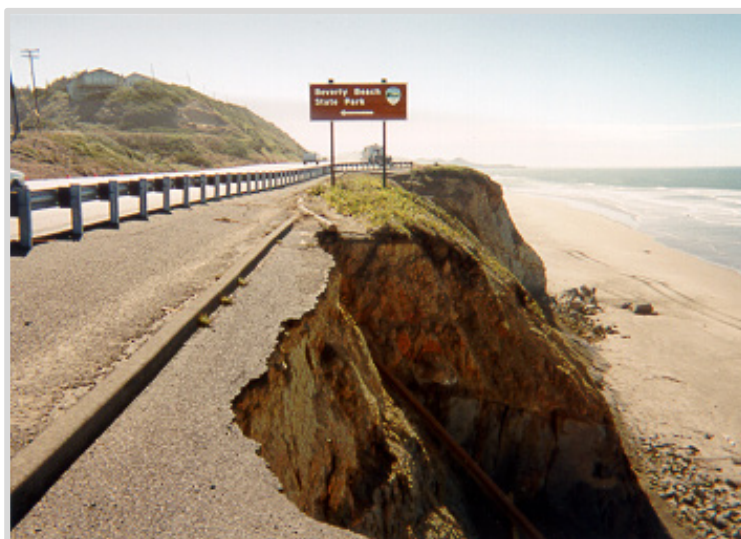
Coastal erosion damage along U.S. 101 at Beverly Beach.
