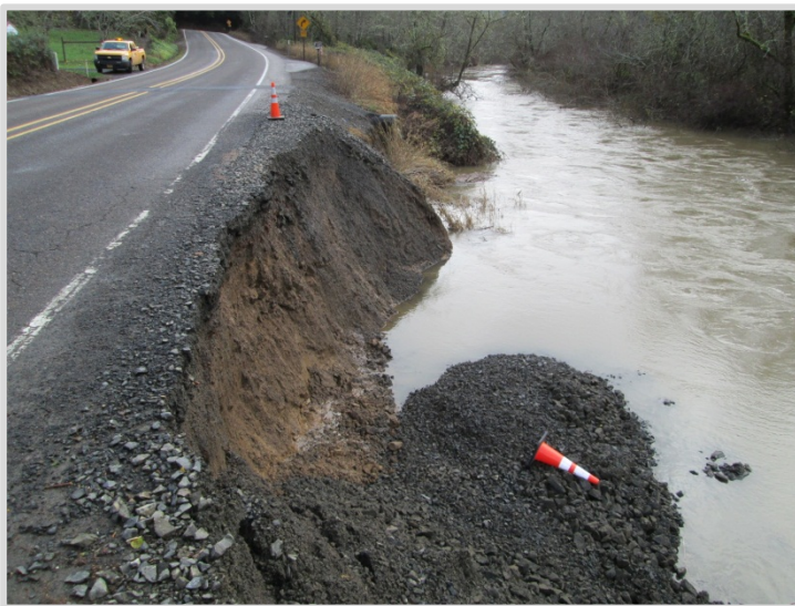
A portion of the highway shoulder on U.S. 20 collapsed into the Yaquina River, December 2012, about 6 miles west of Eddyville in Lincoln County.
