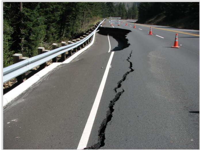
A section of U.S. 101 failed south of Gold Beach after extreme storms in March 2012.
