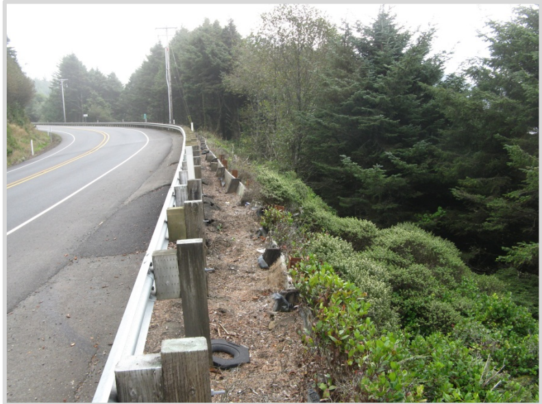
A failing retaining wall on U.S. 101 at the Arch Cape site.
