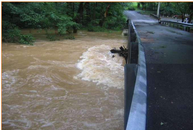
Figure 4-2. Example of Floating Debris Lodged in a Bridge during 2006 Flood Event at Seneca Creek in Germantown, MD
