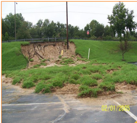
Figure 4-1. Typical Roadway Damage in Maryland
