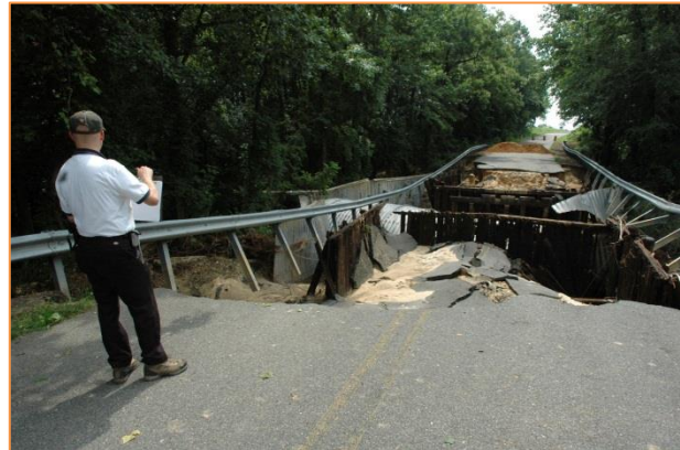
Figure 6-1 Road Failure Caused by Severe Weather Event in Reisterstown, MD Photo source: (FEMA/Skoogfors 2006)
