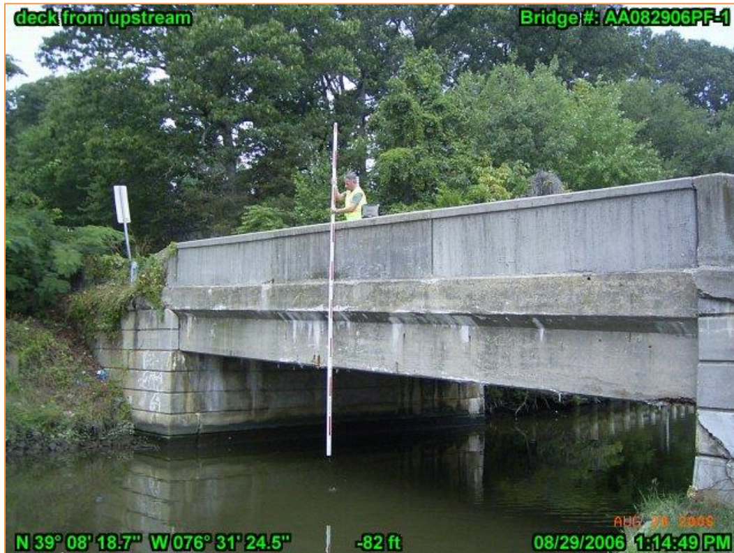
Figure 5-19. Structure 104 Deck from Upstream, Structure 104 is Vulnerable to Sea Level Rise and Storm Surge (VAST 2.6) Photo Source: (Maryland Environmental Services 2006)
