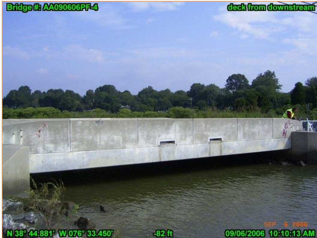
Figure 5-20. Structure 1 Deck from Downstream, Structure 1 is Vulnerable to Changes, Sea Level Rise, and Storm Surge (VAST 2.6) Photo Source: (Maryland Environmental Services 2006)
