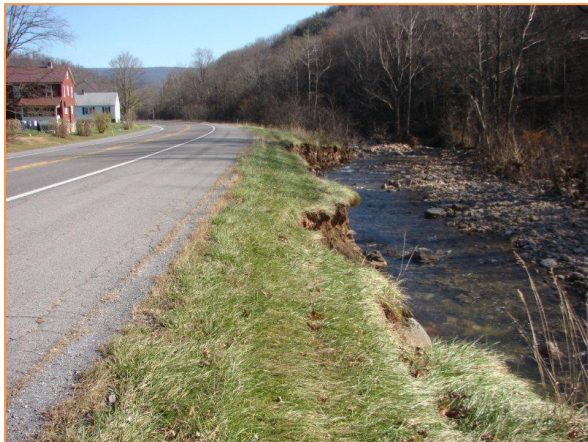
Figure 4-4. Example of roadside erosion along a MD road.
