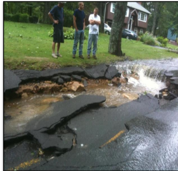
Figure 7 - Damage from Hurricane Irene, Bemis Street, Plymouth Copyright: Foothills Media Group
