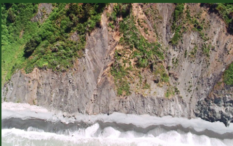
Gully erosion at Last Chance Grade, Del Norte County. Photo credit: Caltrans D1.
