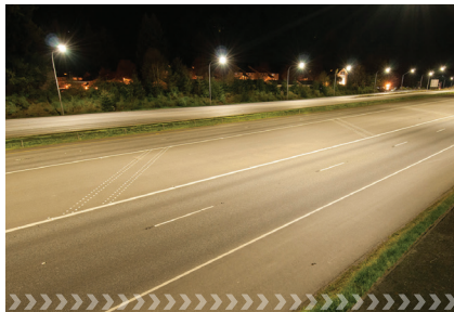
Black Lake Adaptive LED Lighting System on State Highways project | Photo courtesy WSDOT
