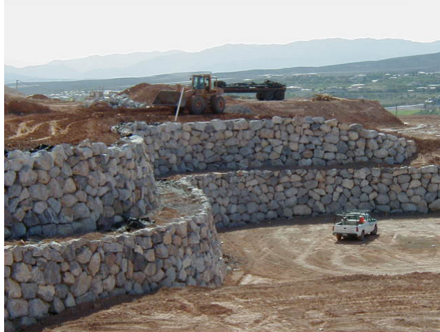
Figure 20. Photograph. “Protecting” rockery used as a facing for a 9.1-m-high (30-ft-high) MSE wall with a 5.5-m (18-ft) maximum tier height in Henderson, Nevada (2001).
