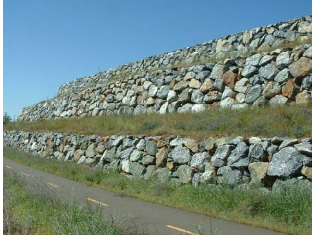
Figure 22. Photograph. Three-tier, 9.1-m-high (30-ft-high) MSE slope with protecting rockery facing, in Folsom, California (2003).
