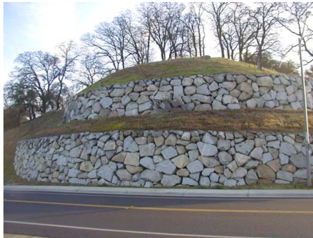
Figure 21. Photograph. “Protecting” rockery used as a facing material for a two-tier, 7.6-m-high (25-ft-high) soil-nail wall in Rocklin, California (1999).
