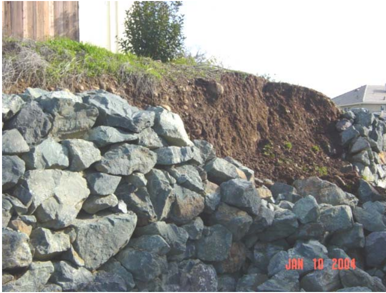
Figure 1. Photograph. Failure of non-engineered rockery in El Dorado Hills, California, 2004.
