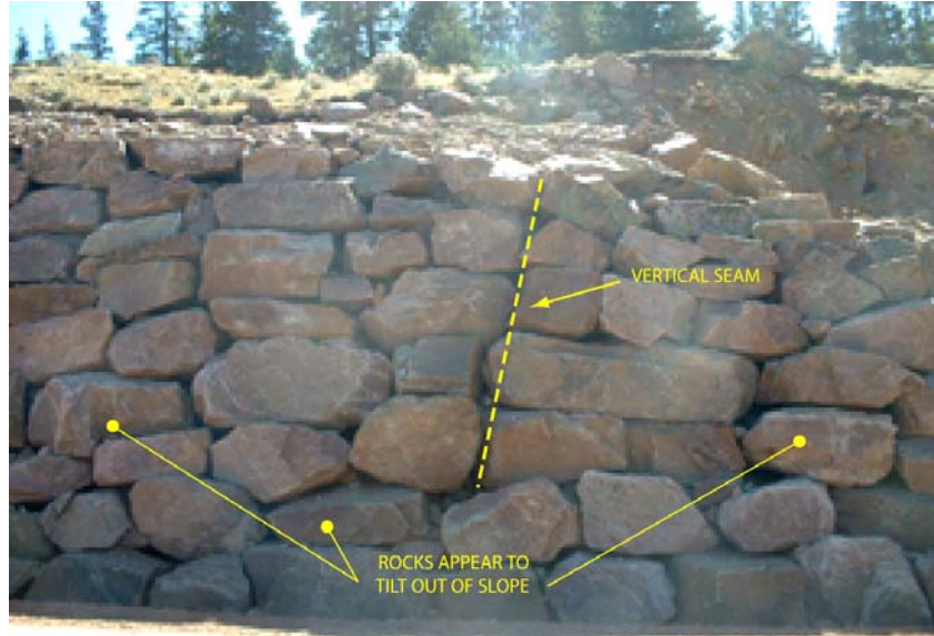
Figure 75. Photograph. Example of improper rockery layout evidences by vertical seams and rocks inclined out of face.
