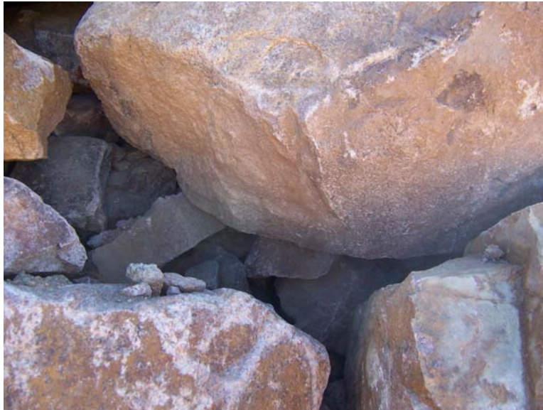
Figure 69. Photograph. Example of improper rock bearing and lack of chinking.
