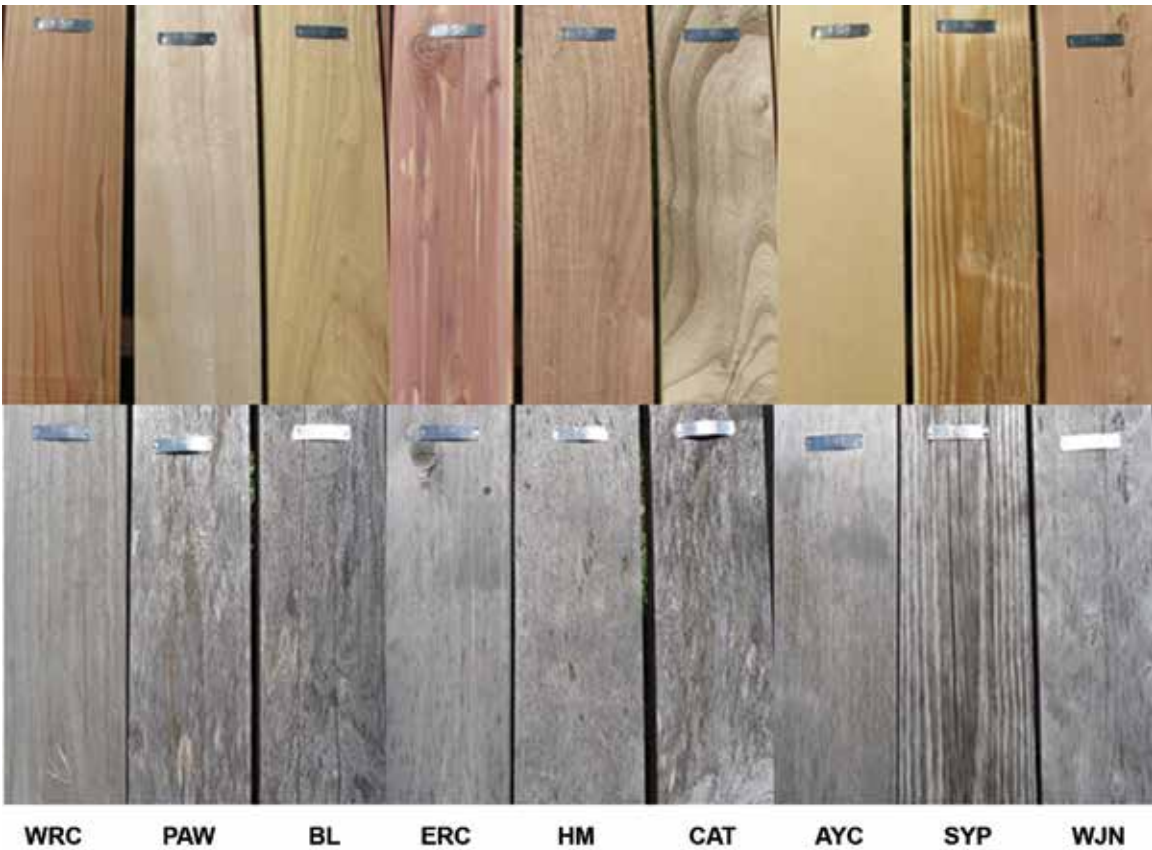
Figure 10. Visual comparison of decking specimens at installation (top row) and after 3 y above-ground exposure at the Valley View test site in Madison, Wisconsin (bottom row). Note the checking of SYP and BL.
